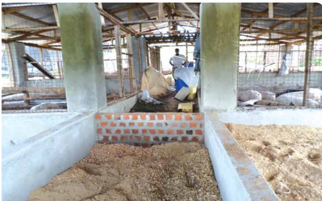
Figure 24 Part of the new extension. In the middle of the forefront is the planned unit for the boar. At the extreme left and right are the units for other pigs
