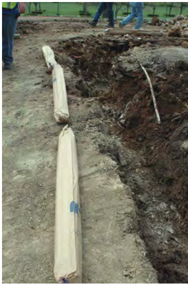
Figure 10a Installing a cathodic protection system on Rumi . Bags of magnesium powder are shown before being placed in the trench around the sculpture.
