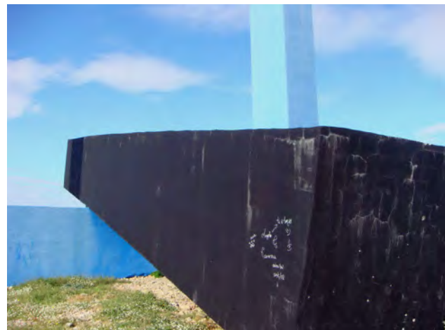
Figure 5 Detail of a work by Tano Festa, showing damage to the black latex paint on concrete from light exposure, rain, and graffiti. Tano Festa, Monumento per un Poeta Morto , 1989 (detail). Situated in Fiumara d'Arte, Sicily. Courtesy Fondazione Fiumara d'Arte. Photo: Tom Learner.
