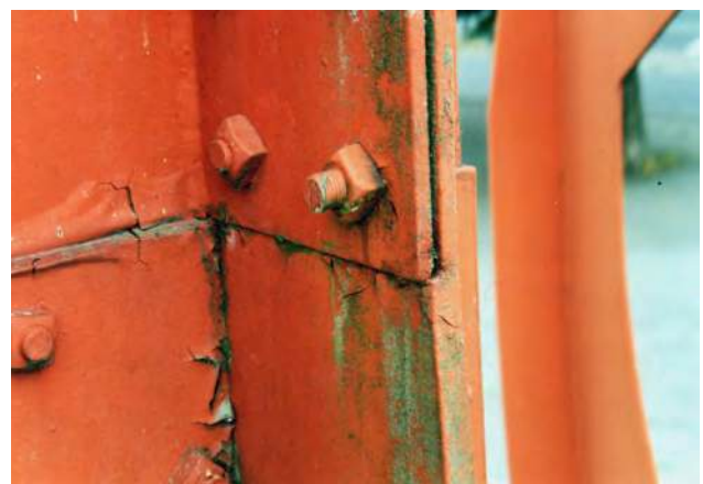
Figure 6 Photo of the west-facing side, showing gaping or open joints where a nut had not been tightly fixed. Loss of paint included flaking of the top layer or several layers, down to the primer. © 2014 Calder Foundation, New York / Artists Rights Society (ARS), New York. © ZMK, Hannover 2003.
