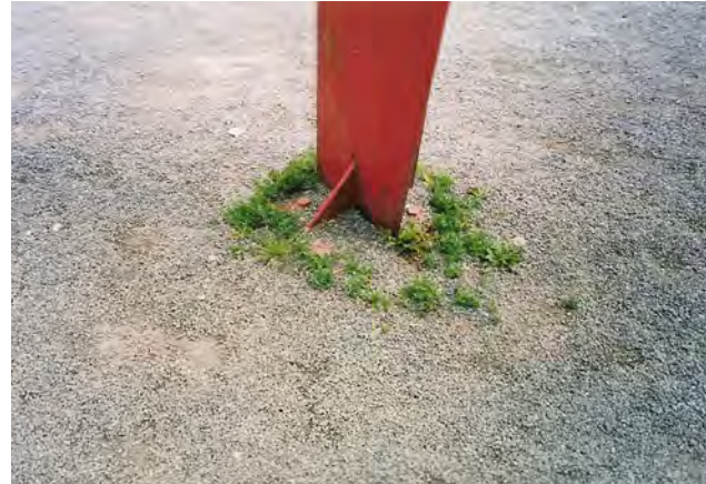
Figure 8 Corrosion damage is evident on the feet of the sculpture, caused by gravel with grass growing over the base plates. © 2014 Calder Foundation, New York / Artists Rights Society (ARS), New York. © ZMK, Hannover 2003.
