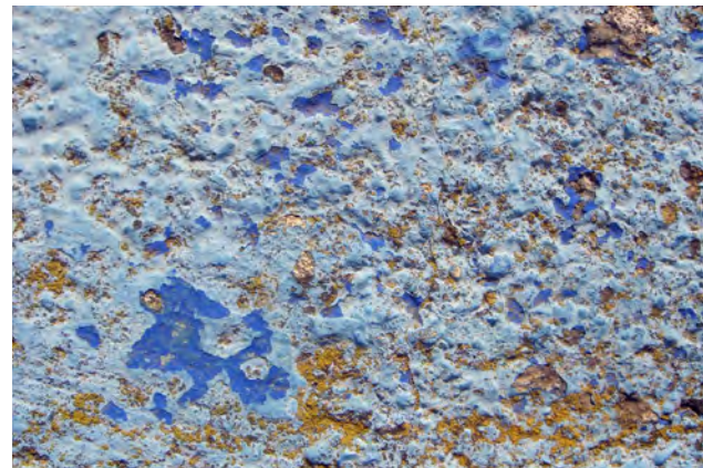
Figure 9 Detail of Energia Mediterranea , showing clear evidence of previous, darker paint layers beneath the existing faded blue, alongside deterioration products of the paint and concrete. Photo: Tom Learner.
