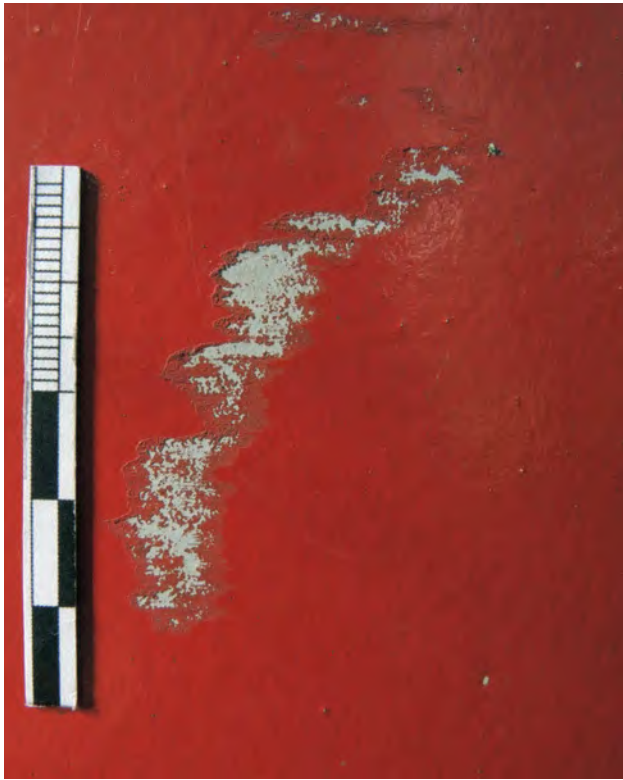
Figure 10 Detail showing damaged paint layer. Photo: Susanne Kensche, 2013.
