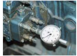
Diesel pump being timed on engine
