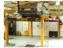
Four post lift in use
