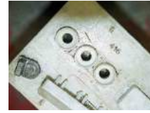
Battery electrolyte level
