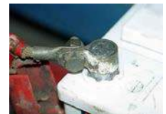
This terminal needs cleaning
