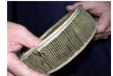
This air filter needs replacing!
