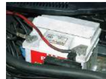
Battery terminals should be...
