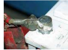
Check terminals for corrosion
