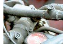
Bleed valves in cooling system
