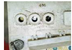
Check battery electrolyte level
