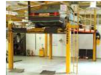
Four post lift in use
