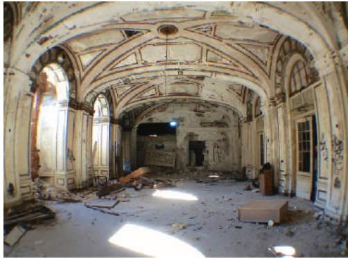
FIGURE 14.6 This photo shows the wreckage of the ballroom at the Lee Plaza Hotel in Detroit, Michigan. Once a landmark, this building is an example of the city’s crumbling infrastructure. (credit: modification of work by Mike Boening)
