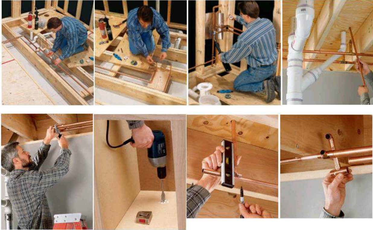
Figure 2.40 Copper pipe system installations
