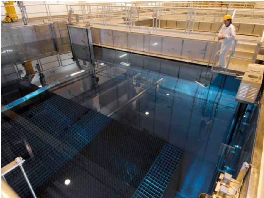
Figure 2-6: Spent fuel storage pool (Source: International Atomic Energy Agency [15])
