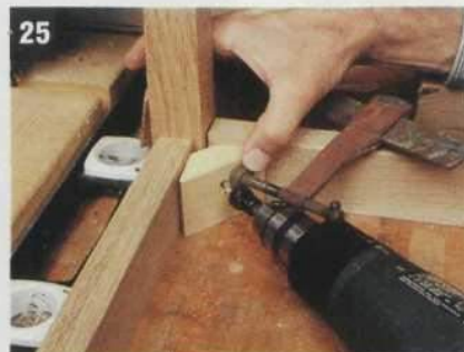
25 Set up the table frame on a flat work surface with a band clamp placed snugly around the frame's circumference. Use a #6 screw bit with the stop collar set at 1¾" to pre-drill a hole through each brace and then into the leg behind it. Center the hole ¾" from the exposed edge, and set the braces flush against the work table.
