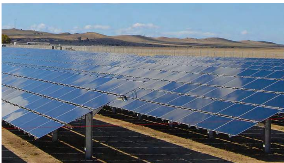
Figure 8.15 Solar cell arrays found in a sunny area converting the solar energy into stored electrical energy. (credit: modification of work by Sarah Swenty, U.S. Fish and Wildlife Service)
