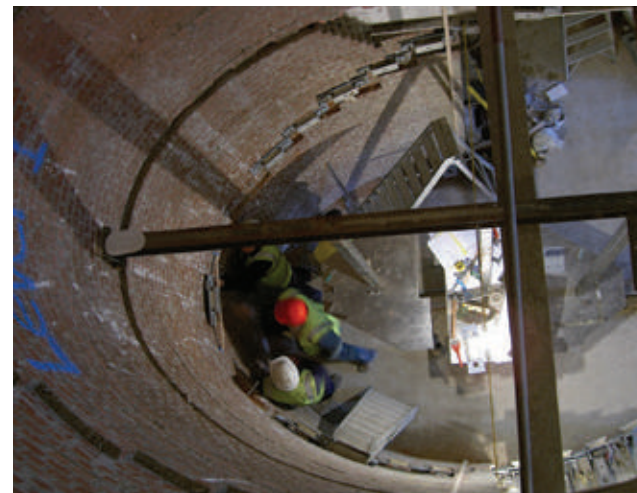
Fig 8.25 The first fix cast aluminium components of the stair in Tudor House being installed in the brick drum of the stair tower
