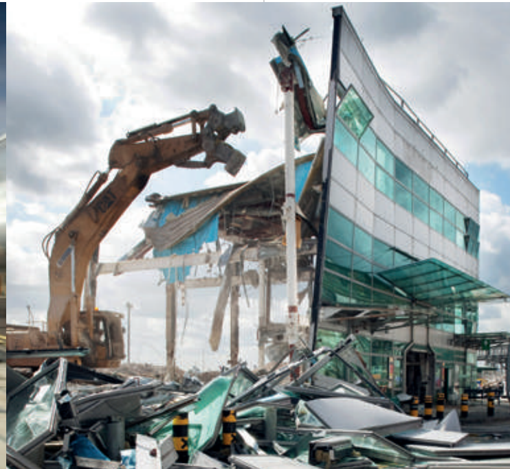
The focus of architects and engineers should shift towards end of life material recovery rather than high-recycled content to improve the environmental impacts of the building and construction sector. Demolition of Heathrow Terminal Two in September 2010.
