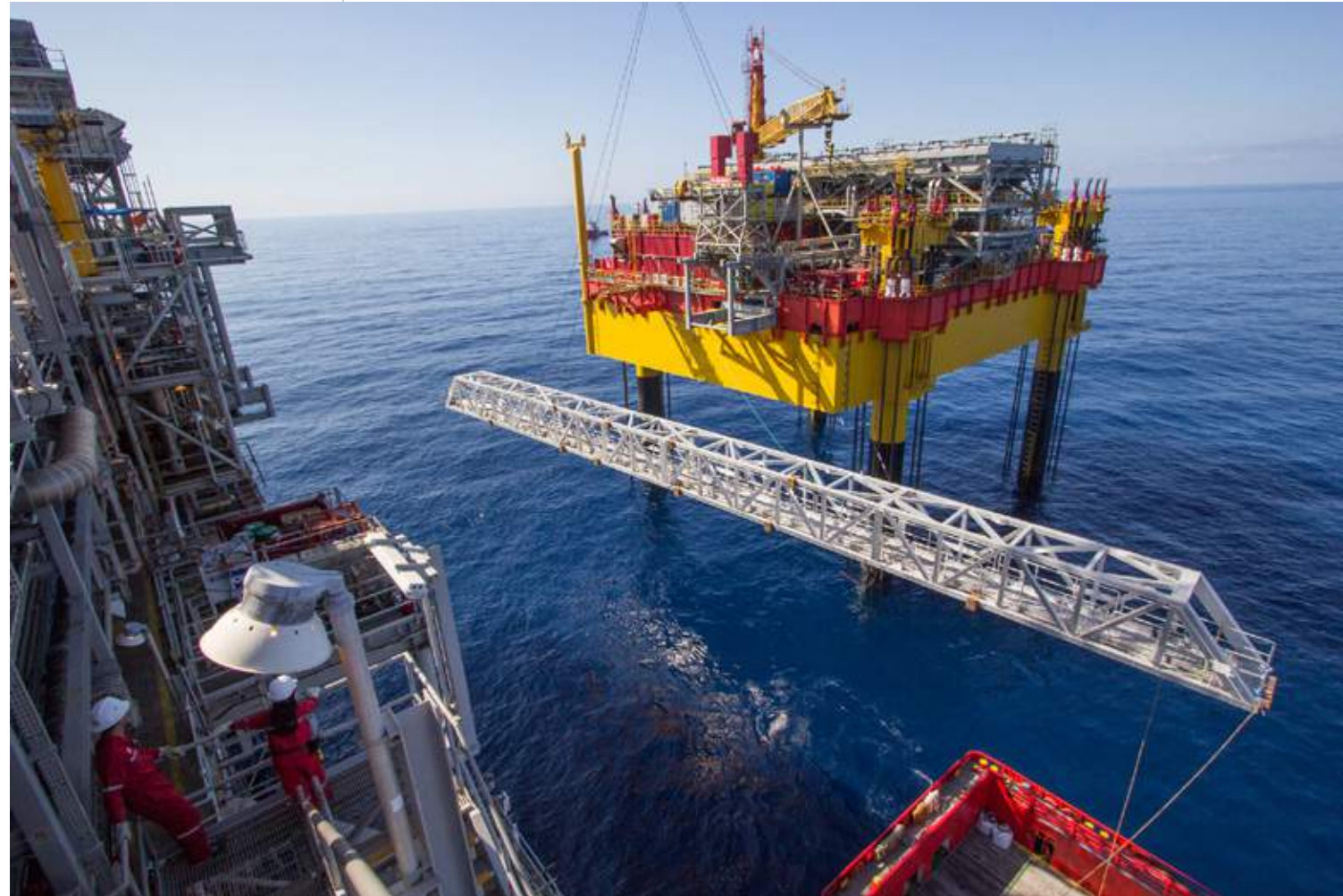
Fig 5.21 46,3m welded aluminium alloy bridge, designed and fabricated by MAADI, being craned into position, 2014, published with permission from the oil extraction company
