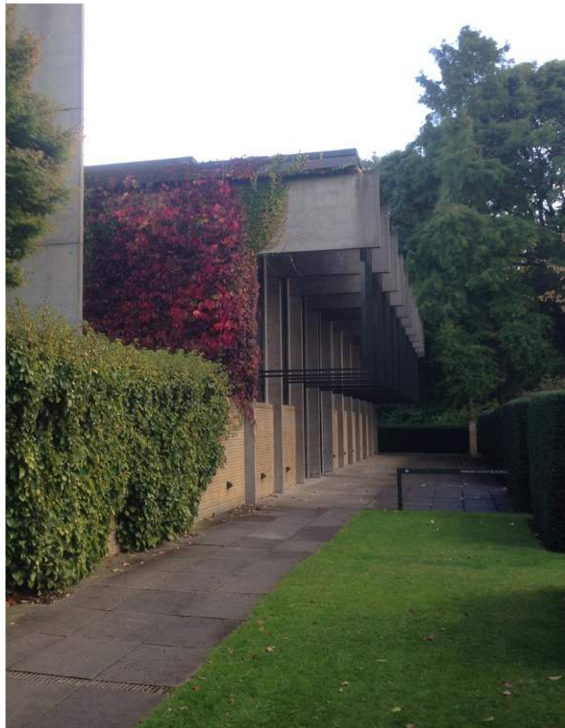
Fig 6.75 Aluminium solar shading of the Grade 1 listed – St Catherine's College, Oxford, England, architect Arne Jacobson, 1964, photographed in 2016
