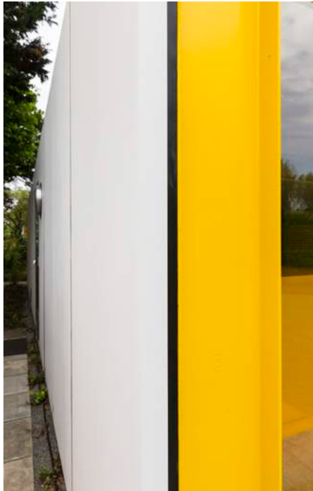
Fig 6.28 Rogers House, 2017, detail of the polyester powder coated aluminium wall panel meeting the painted steel portal frame
