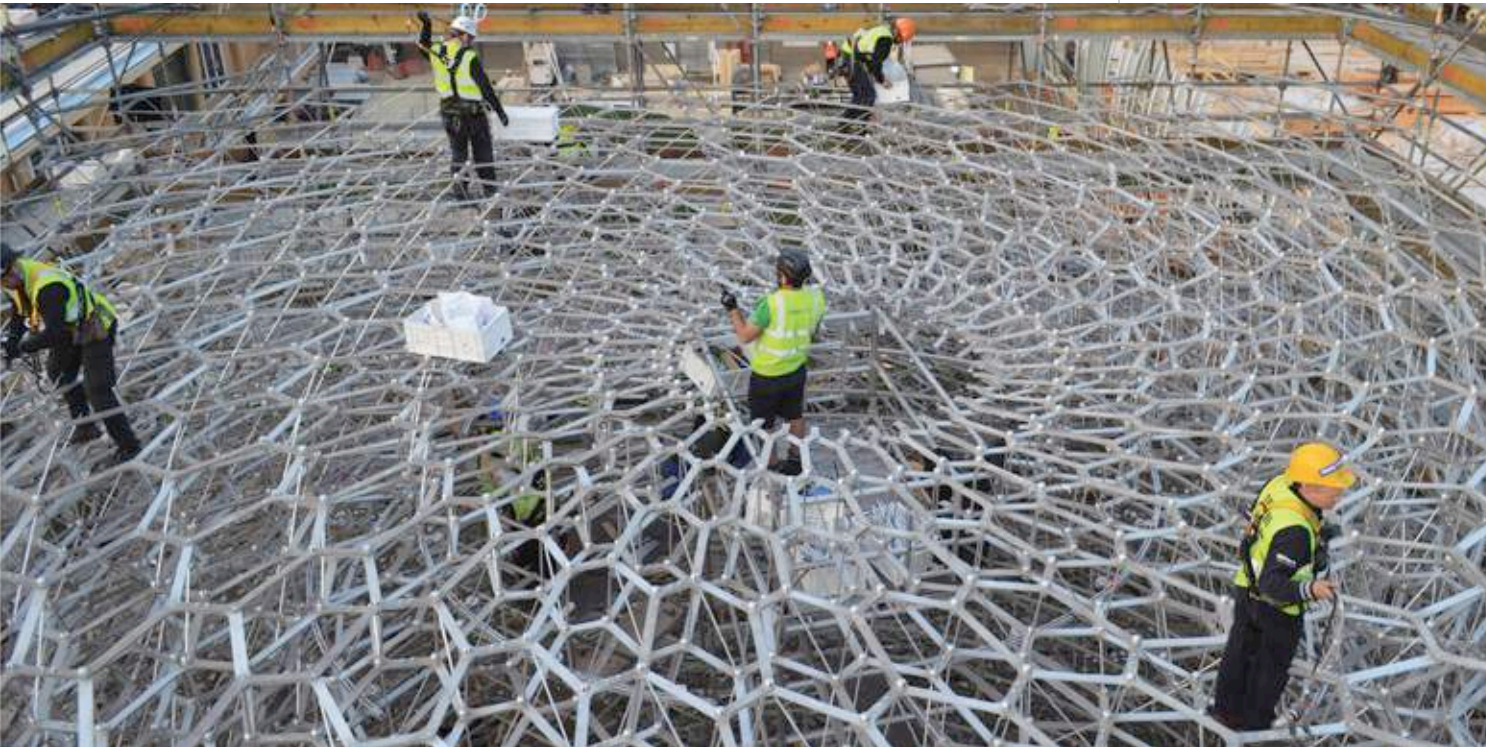
Fig 2.3 The aluminium meshwork of the Hive being assembled by Stage One in Milan, 2015
