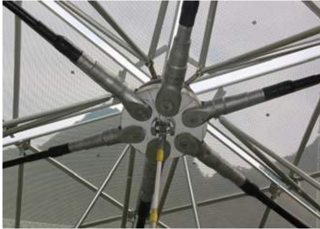
Fig 8.2 Detail of the assembly of The Five Hundred Meter Aperture Spherical Radio Telescope, which is clad in perforated aluminium
