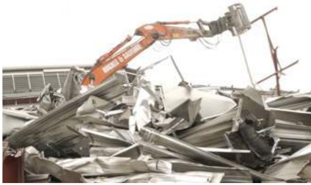
Fig 8.20 Sadly the demolition and recycling of Chetwoods Architects' award winning North Greenwich Sainsbury's was predicted in TSC Book Two Aluminium Recyclability and Recycling , demolition took place in the spring of 2016. An over 99% recycling rate of steel and aluminium was recorded on site by contactors Hughes & Salvidge
