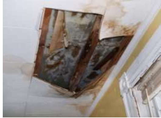
Fig. 75 Roof construction damage by mould
