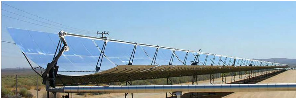
Figure 2.11 Parabolic trough collectors are used to generate electricity in southern California. (credit: “kjkolb”/Wikimedia Commons)
