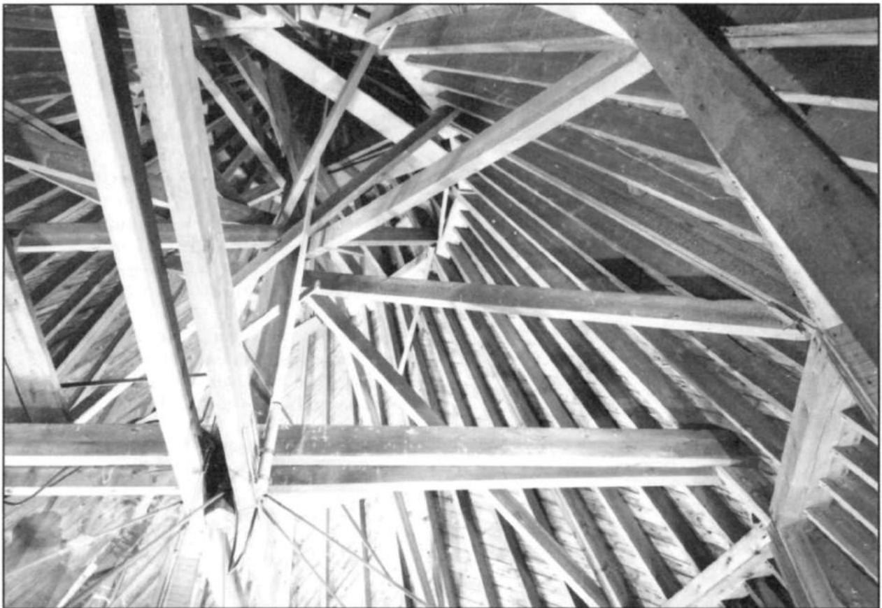
The interior wood framing of the conical roof of the Lawson Water Tower, 1900, in Scituate, Massachusetts. Photo: Jack E. Boucher, HABS Collection.
