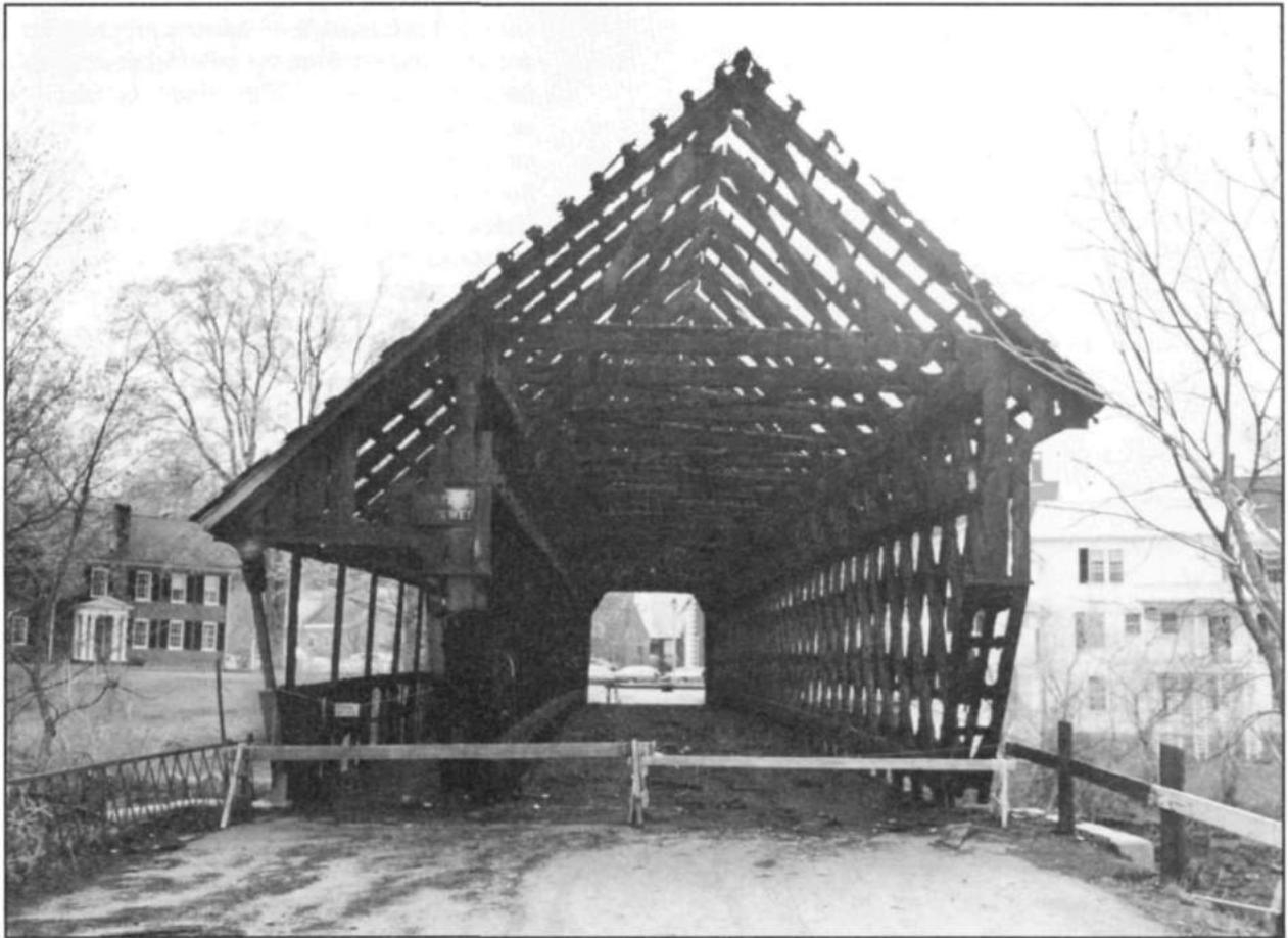
This 19th century, fire-damaged covered bridge reveals the method of cross-braced wood planks used to stabilize the vertical walls. Photo: Hugh T. Henry, Vermont Division of Historic Sites.
