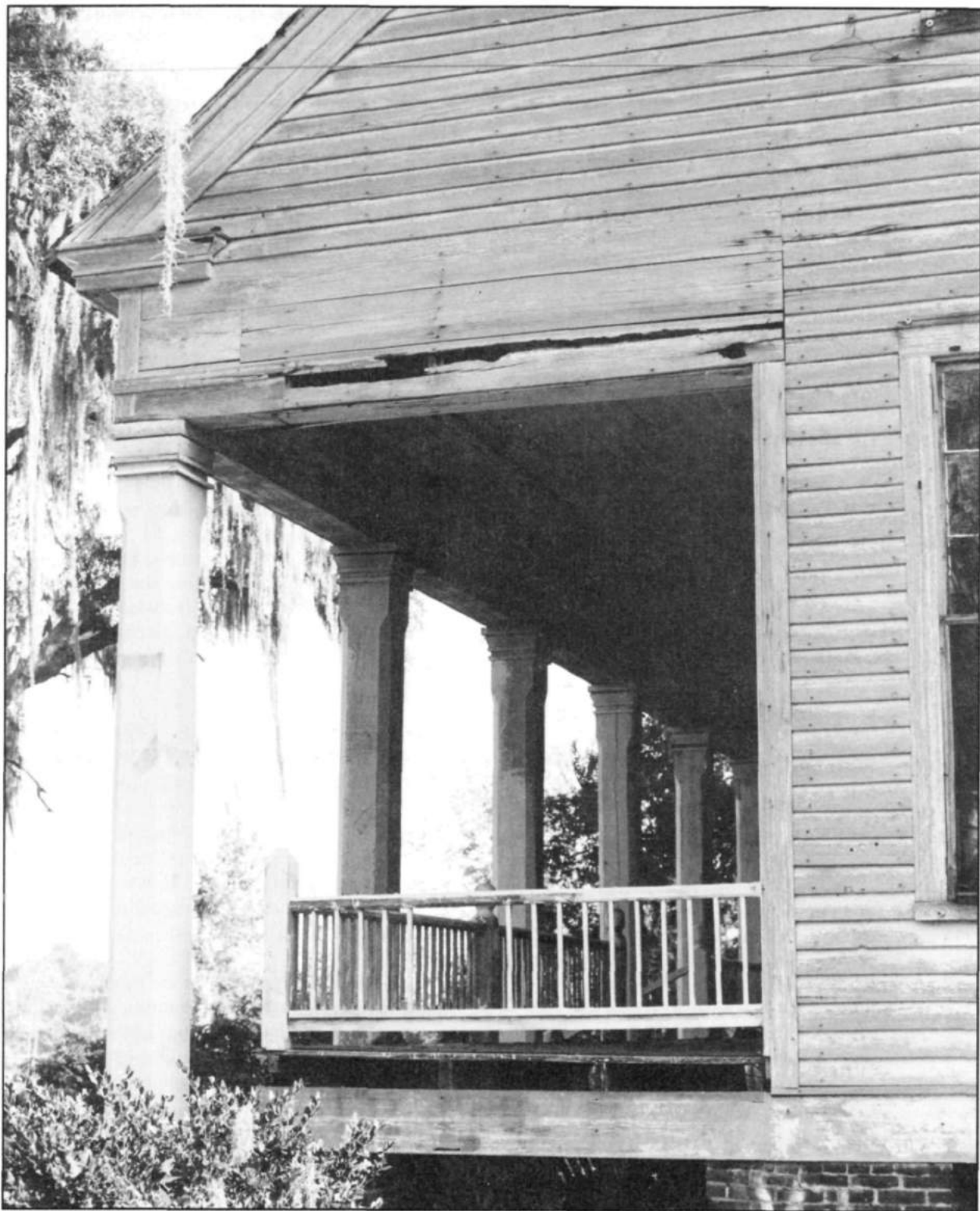
Water damage is evident at the wood cornice return and porch box beam on the Asa May Plantation House, a 19th century antebellum farmhouse in Capps, Florida. Photo: National Park Service files.
