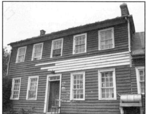
Only those areas of the wood siding that have deteriorated beyond repair should be replaced, as shown here on this wood clapboard house in West Virginia. Photo: Anne Grimmer.
