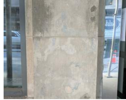
Coating would be appropriate in this case where cleaning revealed staining and previous repairs.
