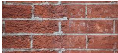
Historic bricks (on the left) damaged by heavy sandblasting.
