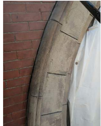
Historic masonry damaged by harsh coating removal and cleaning methods
