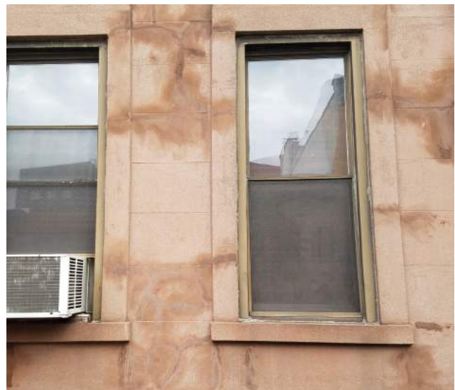
Example of inappropriate coating. Repair mortars and patching compounds should be tinted to match the original material, not the coated and/or stained materials.
