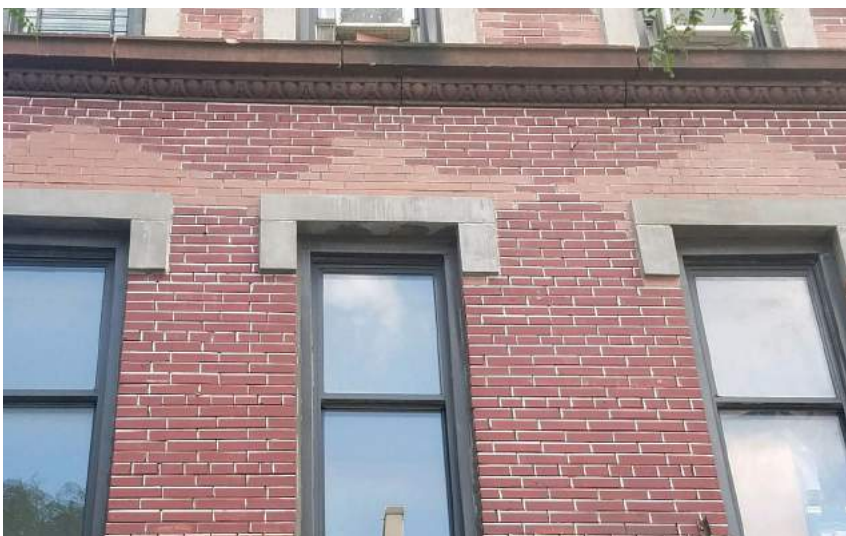
Example of a poor brick match. Note how the new bricks (above the lintels) do not match the historic bricks, calling undue attention to the repair.
