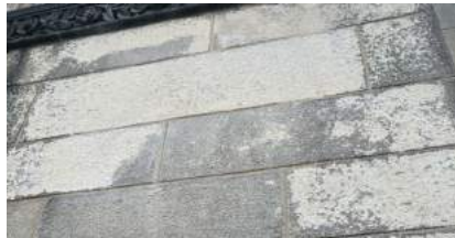
Heavy sandblasting scarred the surface of the masonry, contributing to its deterioration.
