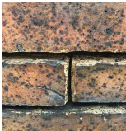
Inappropriate mortar joint removal. Note how the edges of the bricks have been damaged by the process.
