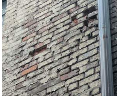
The coating used on the bricks resulted in severe deterioration of the brickwork.
