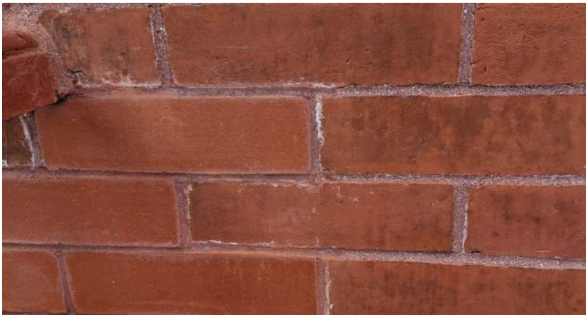
New brick that matches the historic brick in terms of size, dimensions, and finish.
