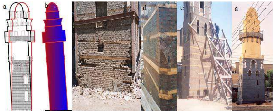
Figure 9. Stabilization the tendencies of the Esna minaret (a, b) architectural documentation (c) the base of the minaret after its tendencies and suffered many problems of damage (d) consolidation of the minaret from the outside by replacement of damaged elements, completion of missed parts and re stitching by wooden beams (e) removal of the steel works after completion of the repair work (f) minaret after restoration and stabilization of tendencies.
