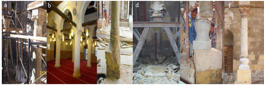
Figure 8. Different applications to restore balance and vertical columns on different types (a, b) re-balancing and vertical columns of bricks for the Abu Hajaj Mosque (c, d, e, f). rebalancing the tendencies of one of the marble columns of the Mosque of Ibn Yarbak.
