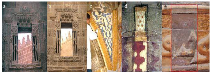
Figure 13. Different applications for the cleaning process (a, b) the upper part of the entrance of Hassan Pasha Taher Complex is characterized by the hollow sculpture of columns (c, d) cleaning of the color composition elements in the Sabil of Ashraf Qaitbay in Sayda Zeinab (e) clean a wood written carving tape.
