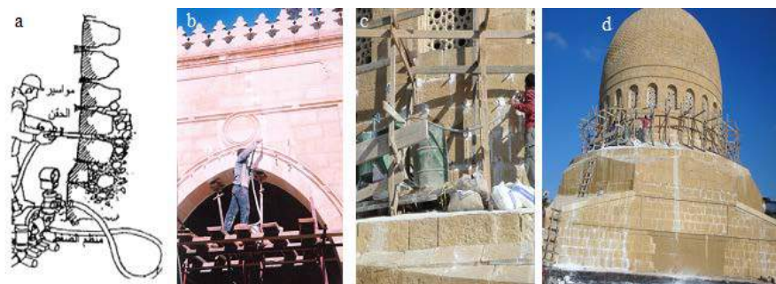
Figure 4. Various applications for injection work in reinforcing the internal fillings and filling gaps in the archaeological buildings (a) Sketch showing injection technique (b) Injection in the arches of the mosque Sayda Soukayna (c, d) Injection for re bonding of Internal filling dome of Ebrahim El Dousouky.
