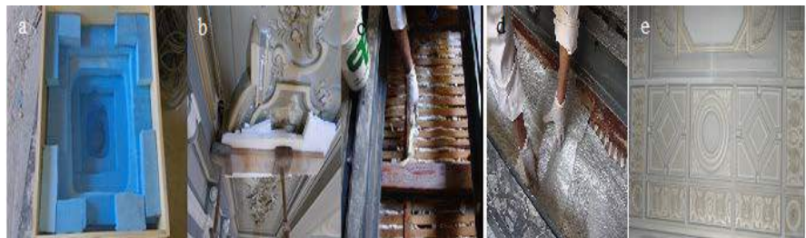
Figure 7. Stages of re construction of the back-support holder from GRP, (a, b) front protection work (c, d) implementation back support holder from GRP (e) decorative ceiling after reinforcement and removal protective layers.
