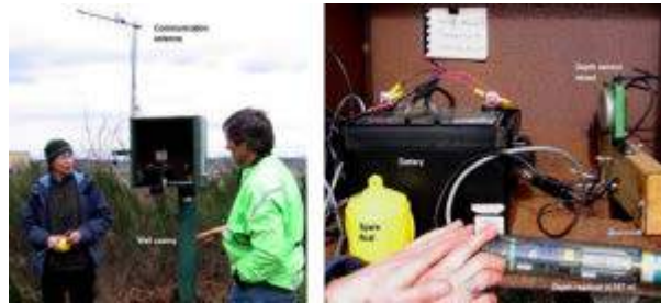
Figure 14.13 B.C. observation well 232 near Cassidy Airport, Vancouver Island. The installation also has a solar panel, which is not visible in this view. [SE]
