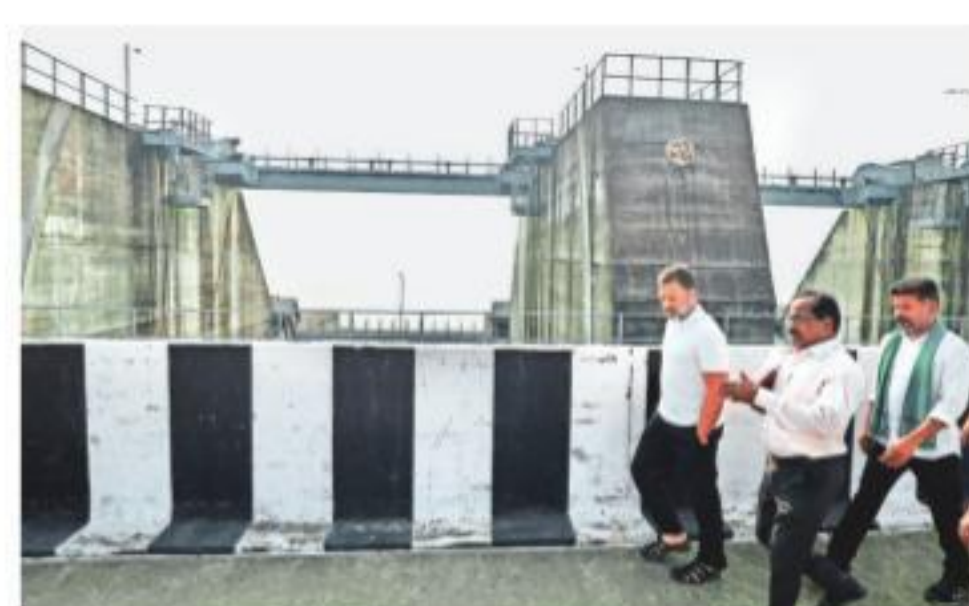
Rahul at the damaged barrage of Kaleshwaram Project, cited as one of the world's largest multi-purpose projects, on Nov 2
