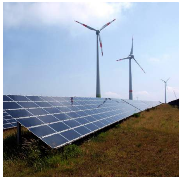
Figure 3: Photograph of Solar Panels and Wind Turbines.
