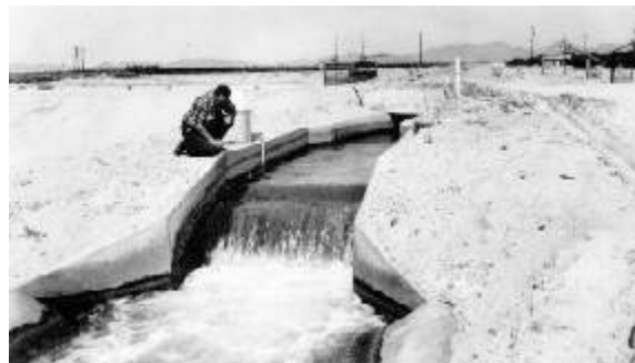
Figure 7-3 -- Suppressed rectangular weir at a canal drop.
