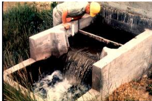
Figure 7-11 -- Weir box turnout with Cipolletti weir.
