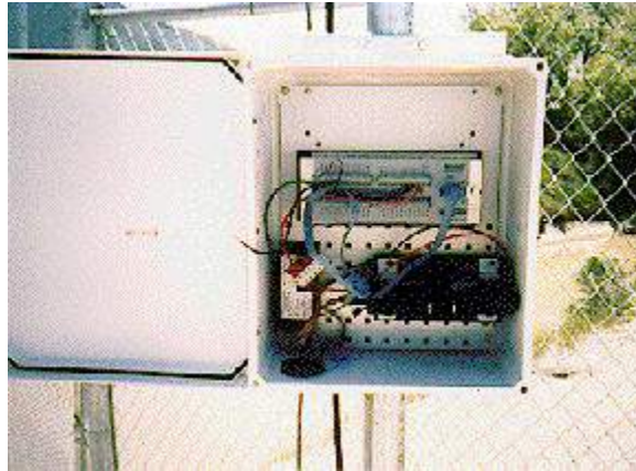
Figure 6-8 -- Programmable battery operated recording unit.
