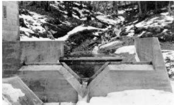
Figure 7-10 -- Compound weir with 90-degree notch and suppressed rectangular crest used by U.S. Forest Service.
