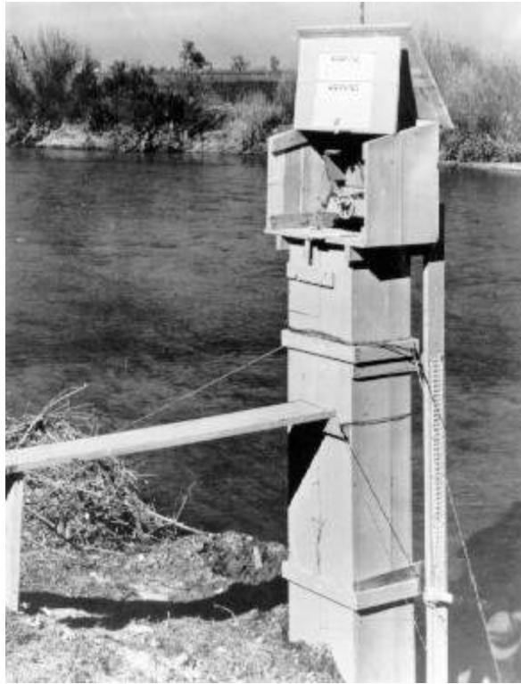
Figure 6-9 -- Stilling well and recorder house made of wood.
