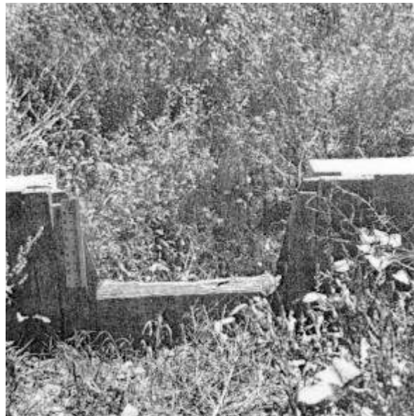
Figure 5-8 -- Poorly maintained weir edge.
