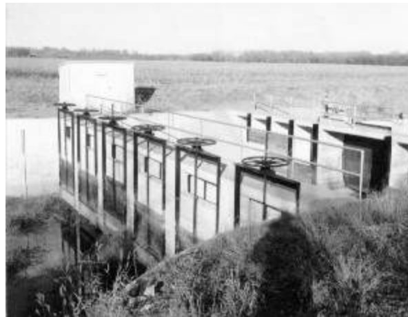
Figure 9-7 -- Gated orifice check structure used to maintain upstream water surface levels and to measure rates of flow in the Courtland Canal, Nebraska.
