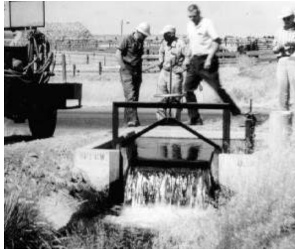
Figure 7-14 -- Adjustable Cipolletti weir in a division box.
