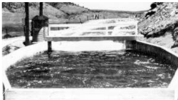
Figure 5-5 -- Underpass-type wave suppressor reduces turbulence and waves in Parshall flumes.
