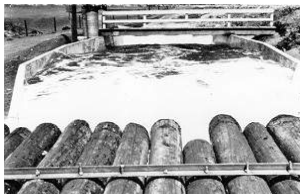
Figure 5-4 -- Turbulence and waves in a Parshall flume produced by an outlet works stilling basin. The log raft failed to quiet the flow.
