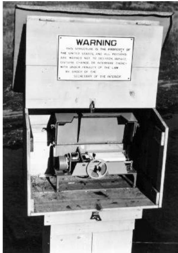
Figure 6-5 -- Typical installation of a continuous water-stage recorder in a wooden shelter.
