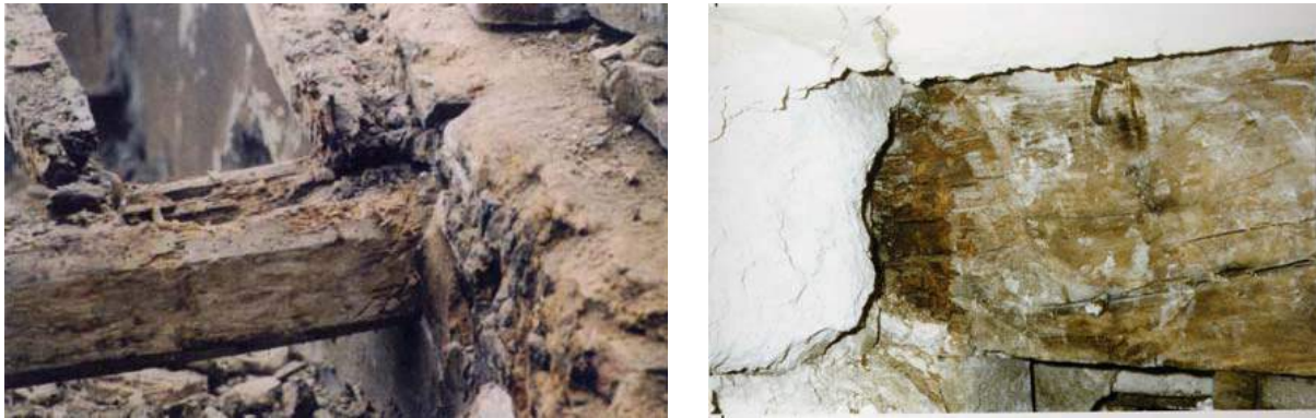
Figure 23 – Wet rot on extremities of beams, in contact with masonry.
