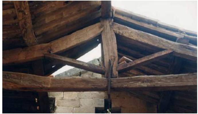
Figure 27 – Church of Mirteto, Italy. Break of the rafter of a truss caused by the instability of the strut.
