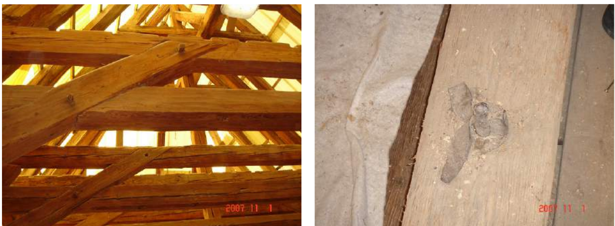
Figure 38 – Detail of halved joints with dowels in a timber roof a connection using metallic elements.
