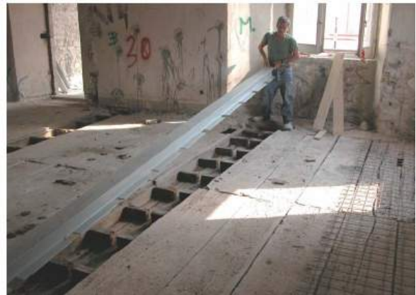
Figure 96 – Strengthening intervention on a beam with an FRP profile mechanically connected to the compression zone of a beam.
