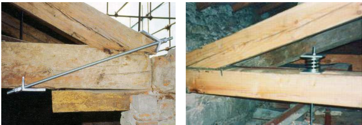
Figure 87 – Repair of connections by moving the location where the tie-beam receives the rafter horizontal thrust.
