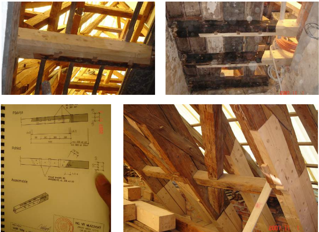
Figure 74 – Prostheticisation with all timber connections and modern carpentry techniques. “Butterfly” dowels joining old floor joists with new strengthening flange beams (Building in Prague).
