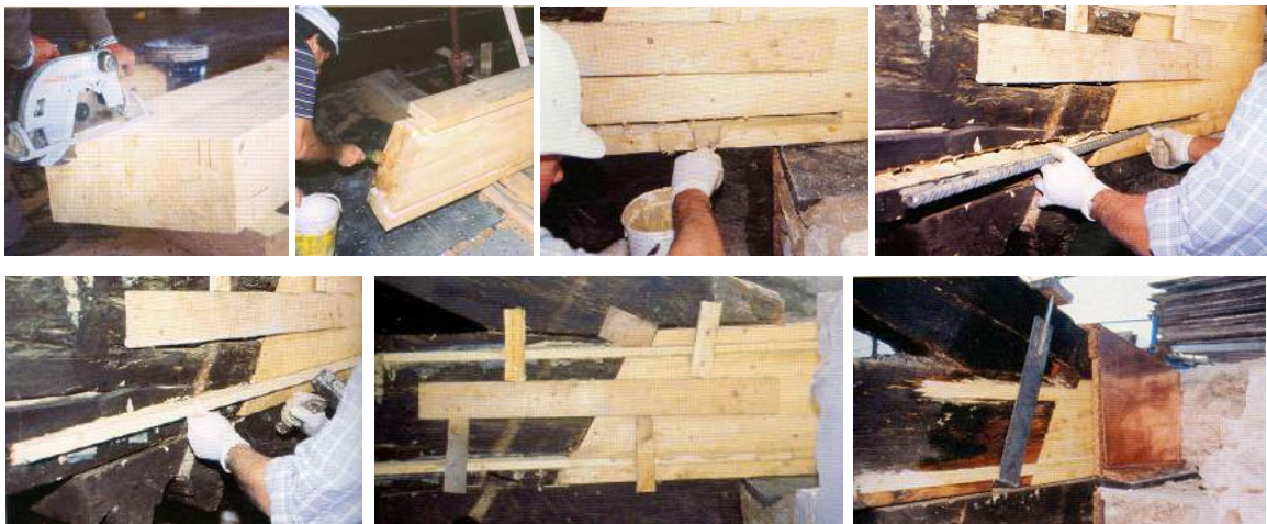
Figure 80 – Sequence of execution of a prosthesisation using steel bonded bars to achieve structural continuity.
