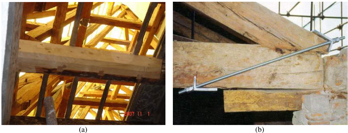
Figure 4 – (a) Prosthesis of a damaged beam extremity by means of timber carpentry, (b) alternative to a prosthesis in the case of a decayed support of a truss.
