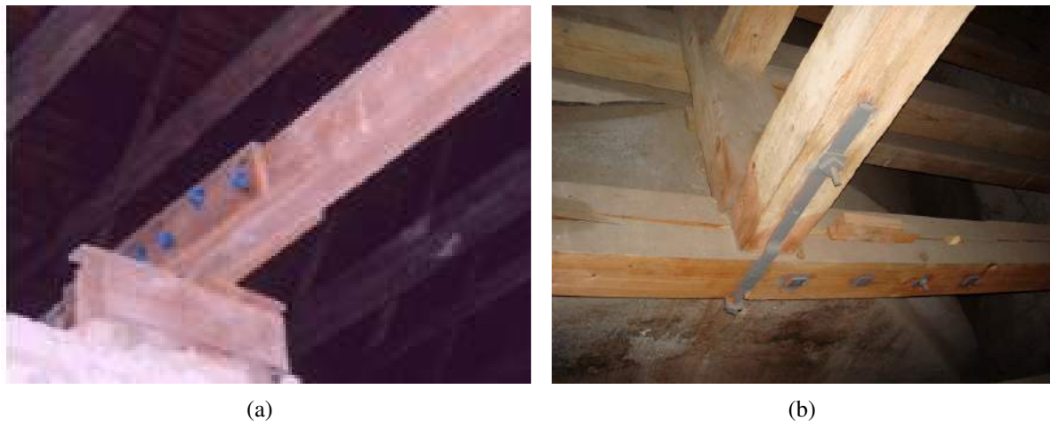
Figure 83 – Example of application of traditional techniques on the repair of cracks. (a) Empalme , (b) Sticking of crack with steel bolts.
