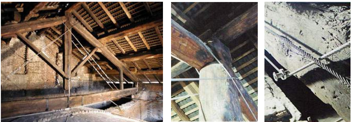
Figure 102 – Scheme and details of an intervention using post-tensioned steel cables and the addition of a timber member, giving the rafters an extra support and loosening the bending on the tie-beam at the same time.
