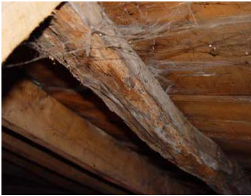
Figure 26 – Reliquary Room of Santa Cruz, Coimbra. Excessive deformation of member.
