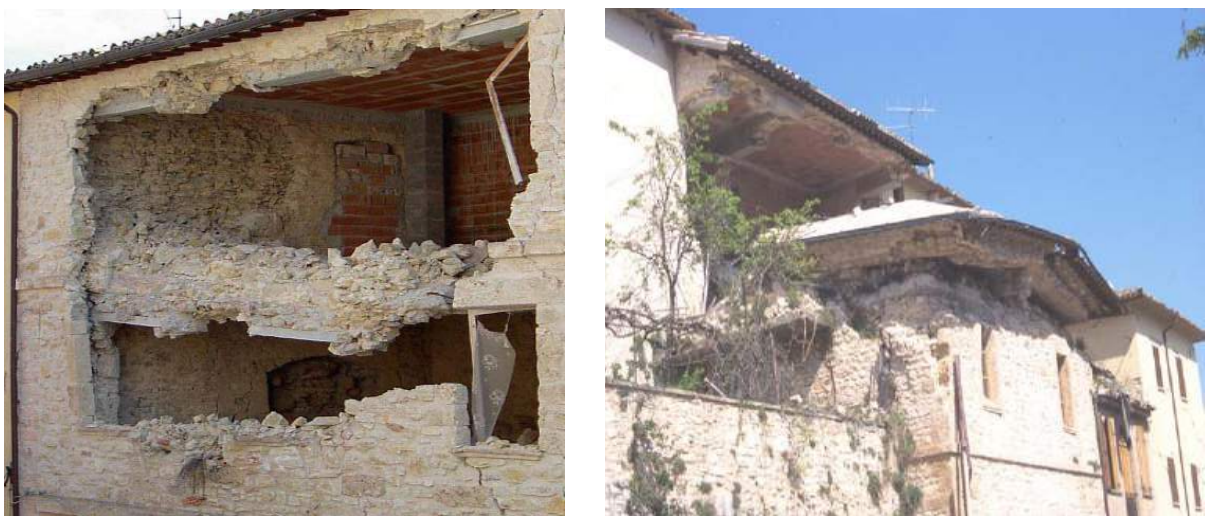
Figure 60 – Out-of-plane collapse of a masonry walls due to “hammering” of concrete floor and roof.
