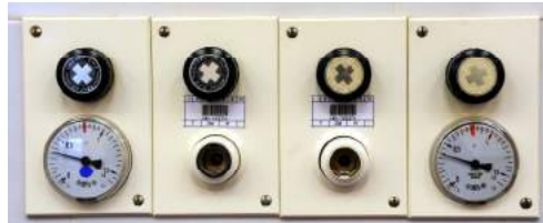
Fig. 16-1 Central oxygen distribution panel
