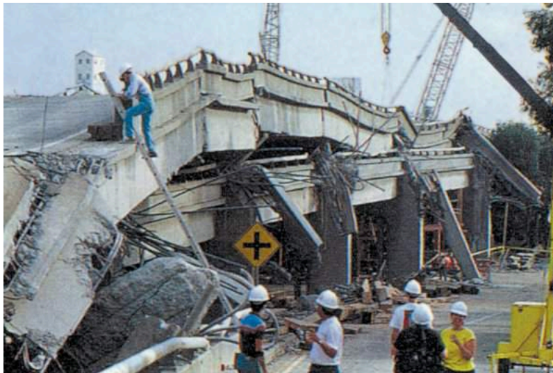
Figure 11.17 A part of the Cypress Freeway in Oakland California that collapsed during the 1989 Loma Prieta earthquake. [from: http://upload.wikimedia.org/wikipedia/commons/9/91/Cypress_collapsed.jpg ]
