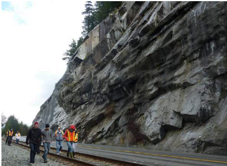
Figure 15.10 Site of the 2008 rock slide at Porteau Cove. Notice the prominent fracture set parallel to the surface of the slope. The slope has been stabilized with rock bolts (top) and holes have been drilled into the rock to improve drainage (one is visible in the lower right). Risk to passing vehicles from rock fall has been reduced by hanging mesh curtains (background). [SE photo 2012]
