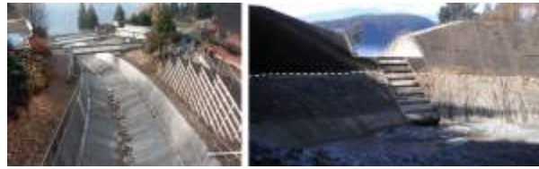
Figure 15.22 Two strategies for mitigating debris flows on the Sea-to-Sky Highway. Left: A concrete-lined channel on Alberta Creek allows debris to flow quickly through to the ocean. Right: A debris-flow catchment basin on Charles Creek. In 2010, a debris flow filled the basin to the level of the dotted white line. [SE]
