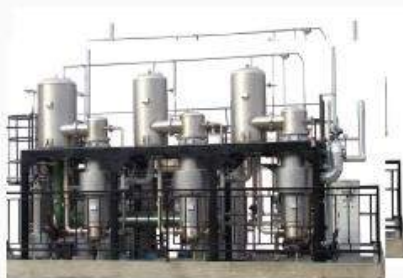
3-stage caustic soda recovery plant
