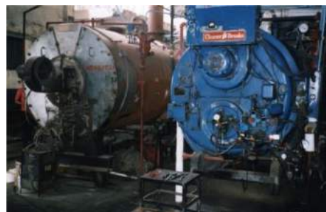
Figure 4-20: Fuel oil operated boilers [87]
