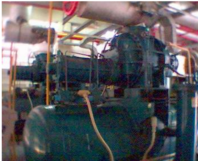
Figura 2.04 - Compressor parafuso Frick RWB-II 301,8 kW. (Mod. TDSH 233S 2334E). (-10/+35°C)
