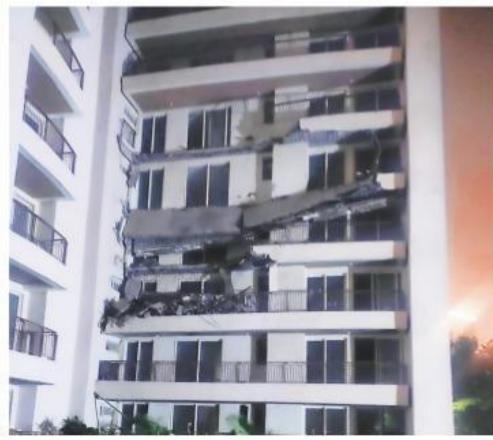
On November 9, four balconies had collapsed in Tower D. No casualty was reported as the tower was already vacant. Express
