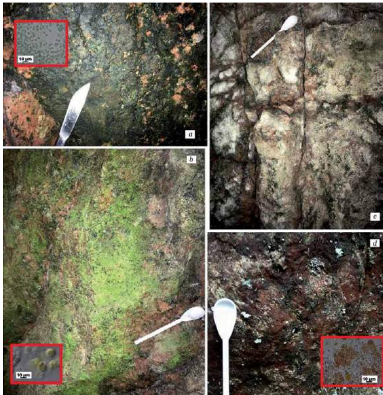
Figure 2. Different types of biofilms and deposits in the Vyborg tunnels.
