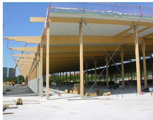
Glulam hall under construction. Permanent cross bracing at a gable wall transfers horizontal loading from stiff roof sheet to the ground
