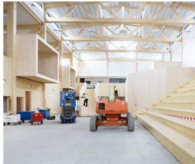
Scissor lift and boom lift during assembly of glulam and CLT frame of a school building, Skellefteå.
