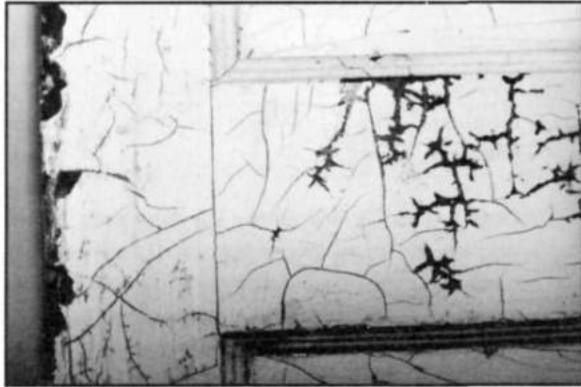
Checking of paint on this interior door surface has developed due to a loss of elasticity in the top layer of paint. Photo: National Park Service files.
