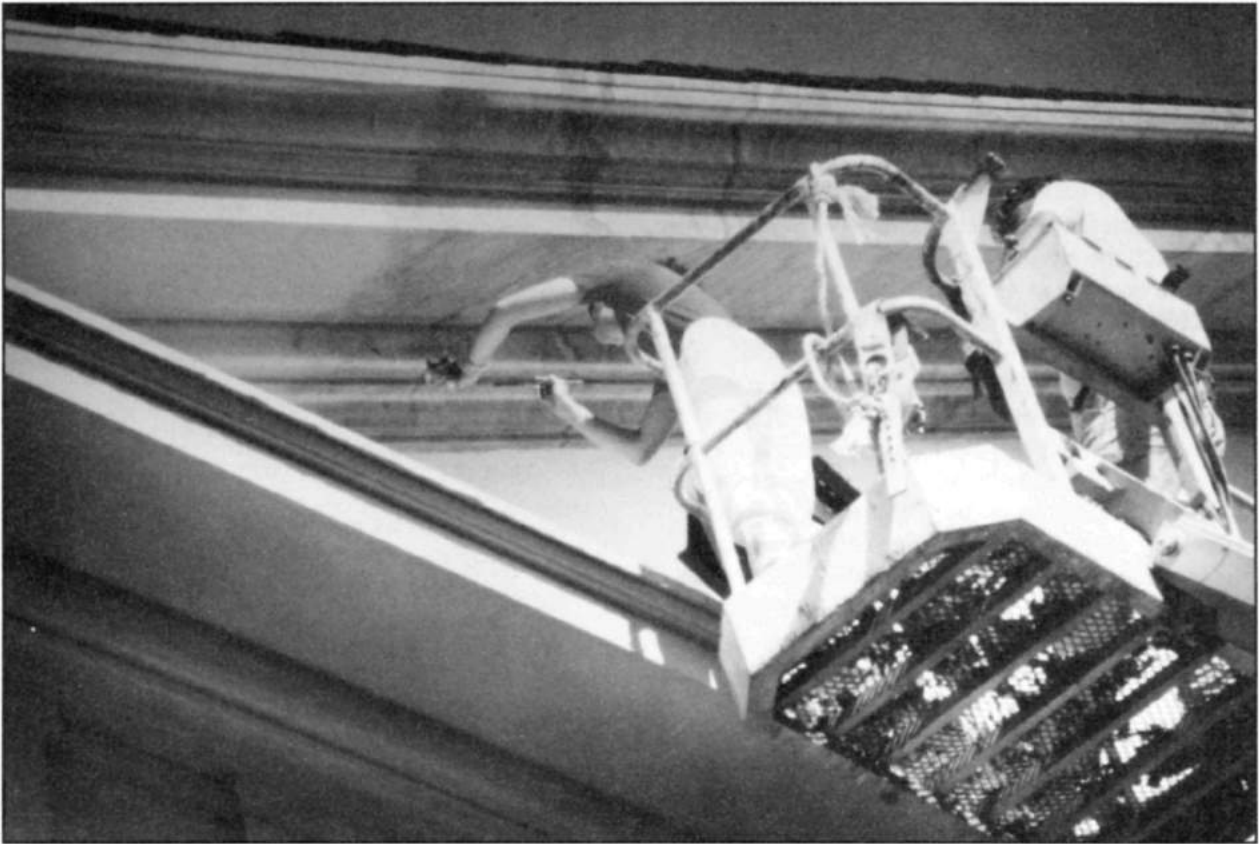
Museum technicians engaged in recreating c. 1860s marbling on the stucco surface of Arlington House, Arlington, Virginia, an early 19th century mansion. Photo: George Siekinen.
