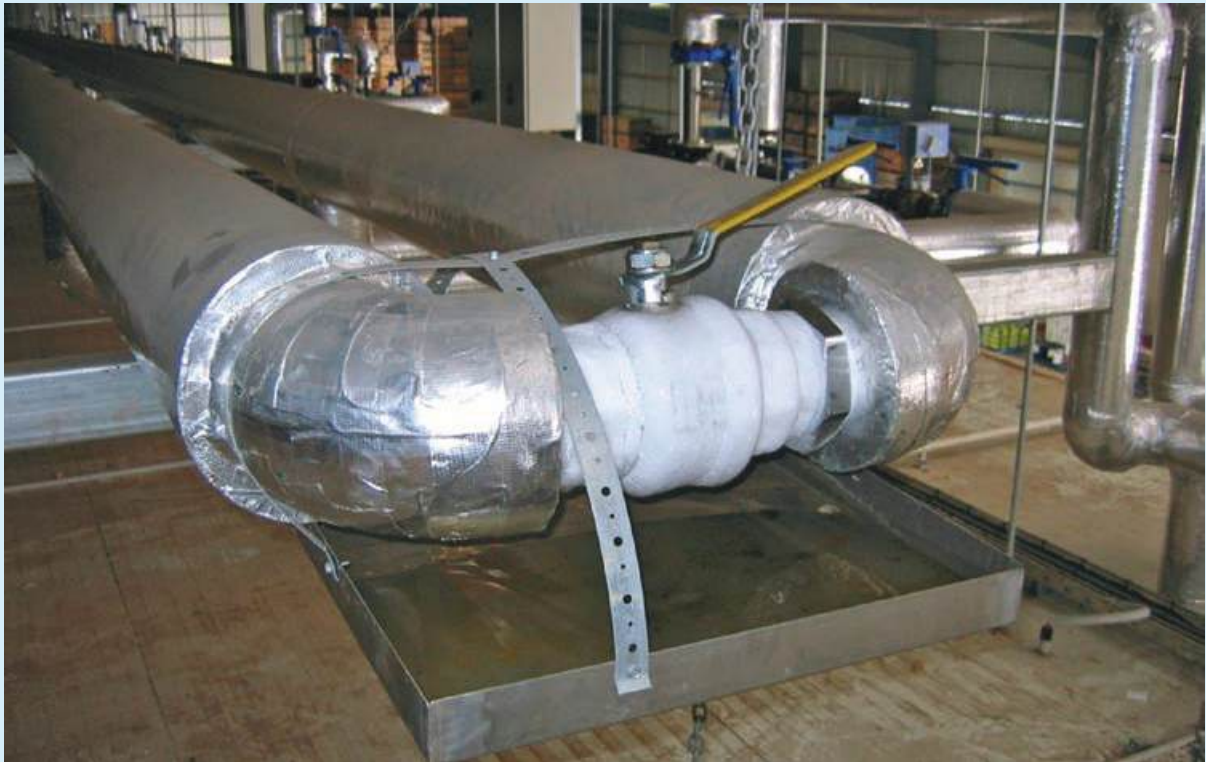
Figure 38: Before: a fully opened ball valve at the end of the circuit to bypass unused flow
