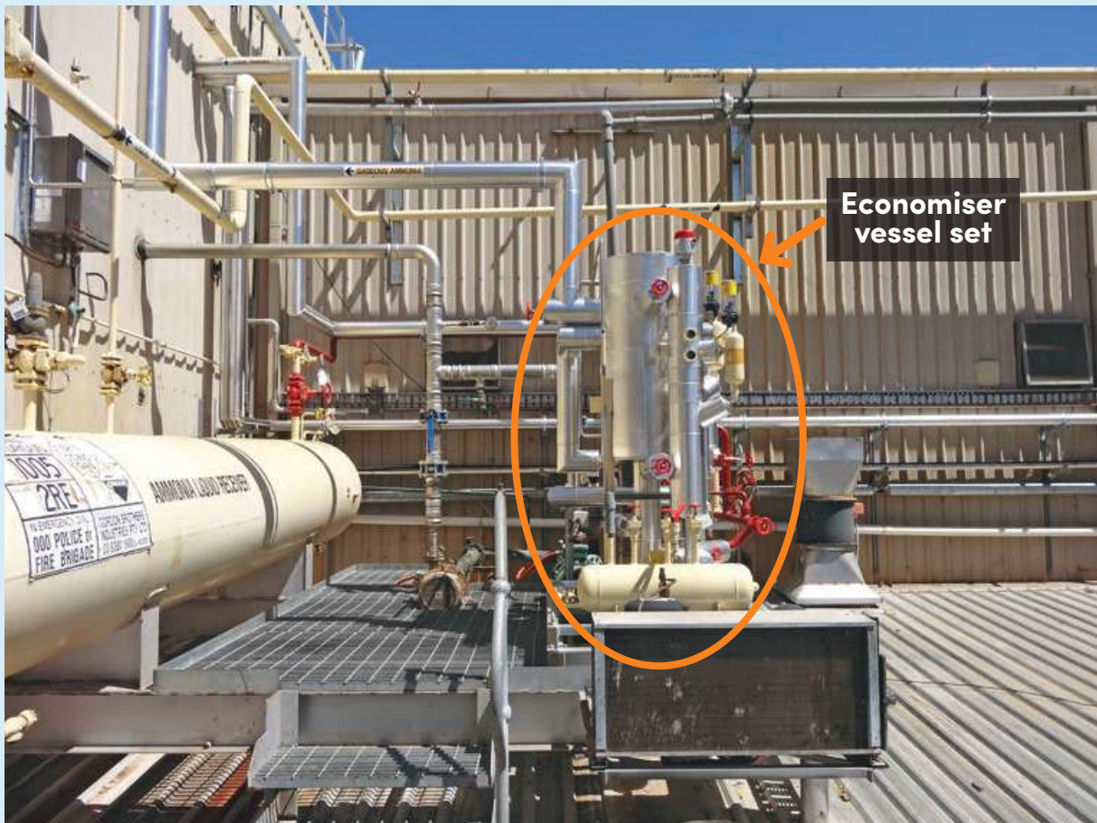
Figure 24: Rivalea's economiser vessel set for condensate sub-cooling
