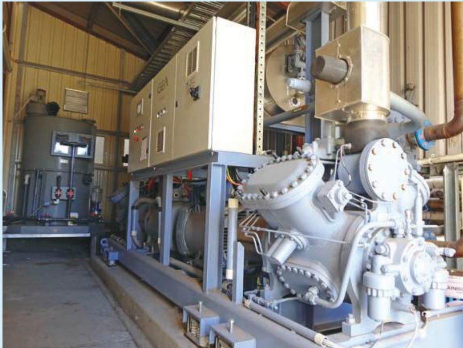
Figure 33: Water-cooled ammonia chiller at Riverina Fresh, Wagga Wagga
