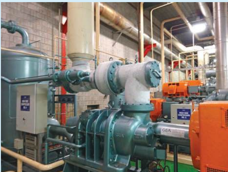
Figure 32: Plant room at Simplot Ulverstone
