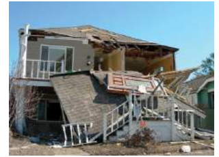
Figure 6.2 Hurricane Katrina Aftermath
