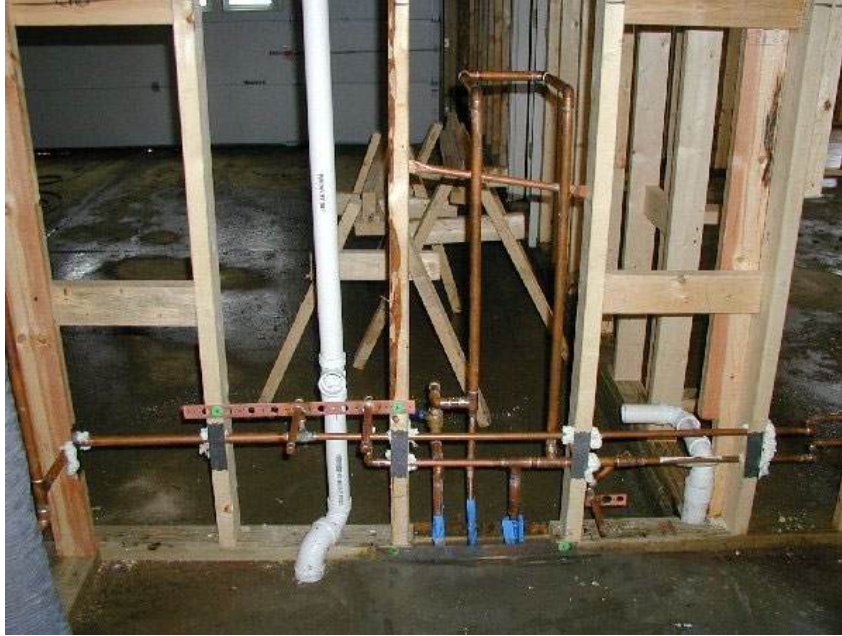
Lavatory or bathroom set-up with a Dirty Arm and possible water softener loop.
