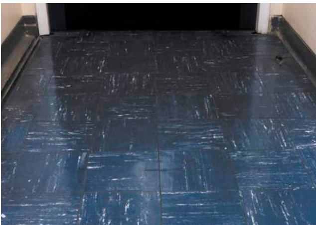
Figure 48e Asbestos-containing vinyl floor tiles
