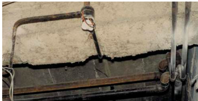
Figure 48b Poorly tamped sprayed chrysotile fireproofing on a structural steel beam holding up a concrete floor, showing some overspray onto the concrete and damage by electrical work
