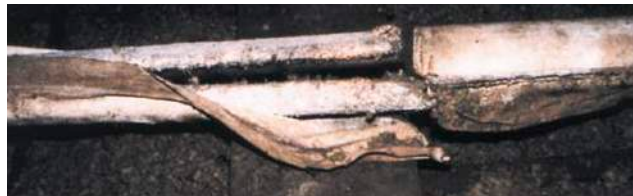
Figure 48a Asbestos-insulated water pipes showing evidence of maintenance work damage, with detached preformed sections and calico wrapping
