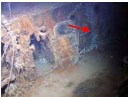
Recreation space/heads, Forecastle deck (forward - starboard). This photograph shows the boundary between the burnt and unburnt bulkhead (see arrow).
