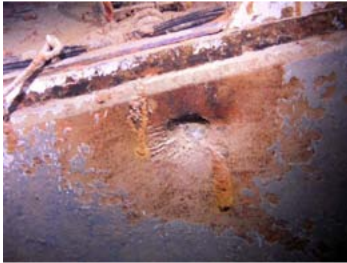
Figure 240: Example of shell damage that probably sprayed hot fragments over the surrounding deck [311]
