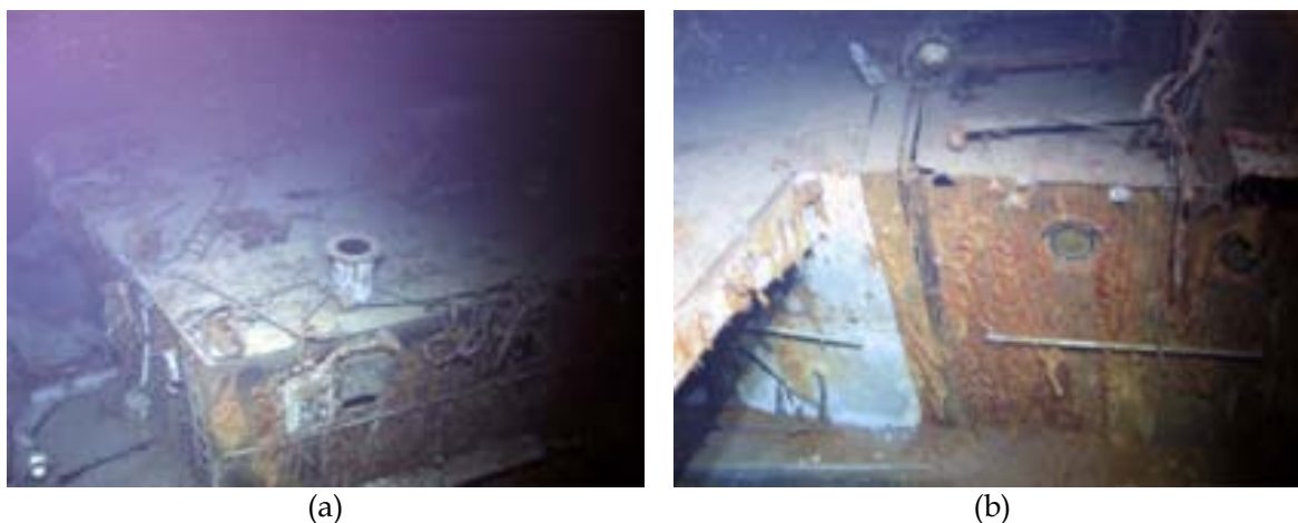
Figure 258- Fire damage to the port side aft upper deck in the vicinity of the 4" gun deck [254, 312]
