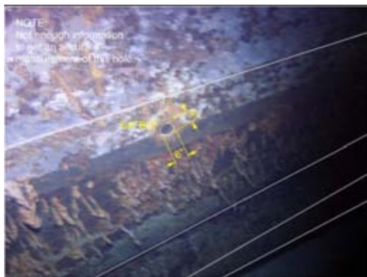
Figure 335: In vicinity of Refrigerating Machinery Compartment, Platform deck [370]
