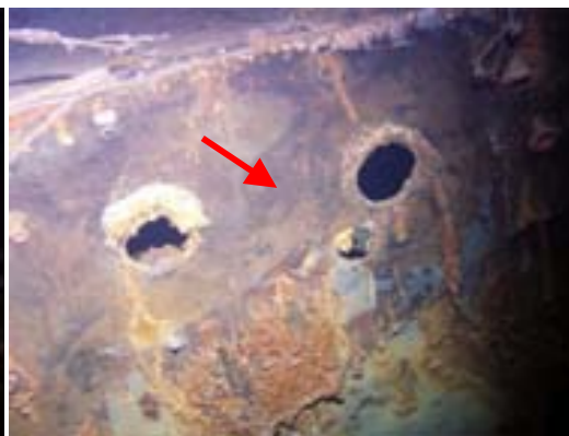
Canteen / dispensary, upper deck (forward - starboard). Note the blackened paint and the corrosion where the paint has been removed.
