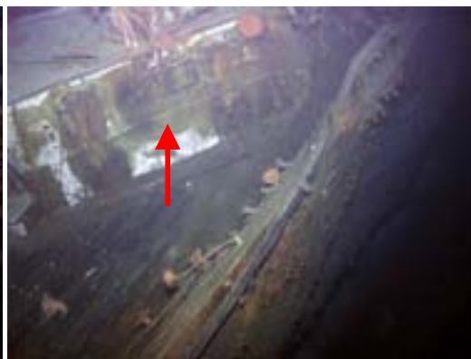
Captain's sleeping space, upper deck (aft - starboard). Note the discoloured patches due to heat transfer from a fire (see arrow).
