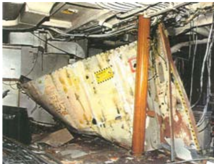
Figure 257: Damage to a bulkhead from the internal blast from a 4.75 kg cased charge [285]
