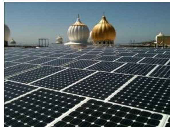
434kW system in San Jose, CA
