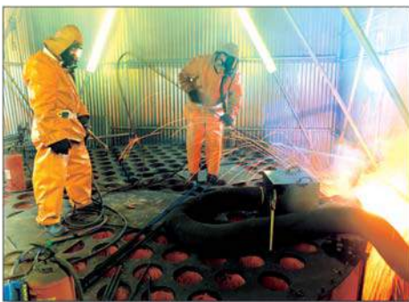
Top biological shield being dismantled using a thermic lance process at the Windscale Advanced Gas-cooled Reactor Dismantling Project.
