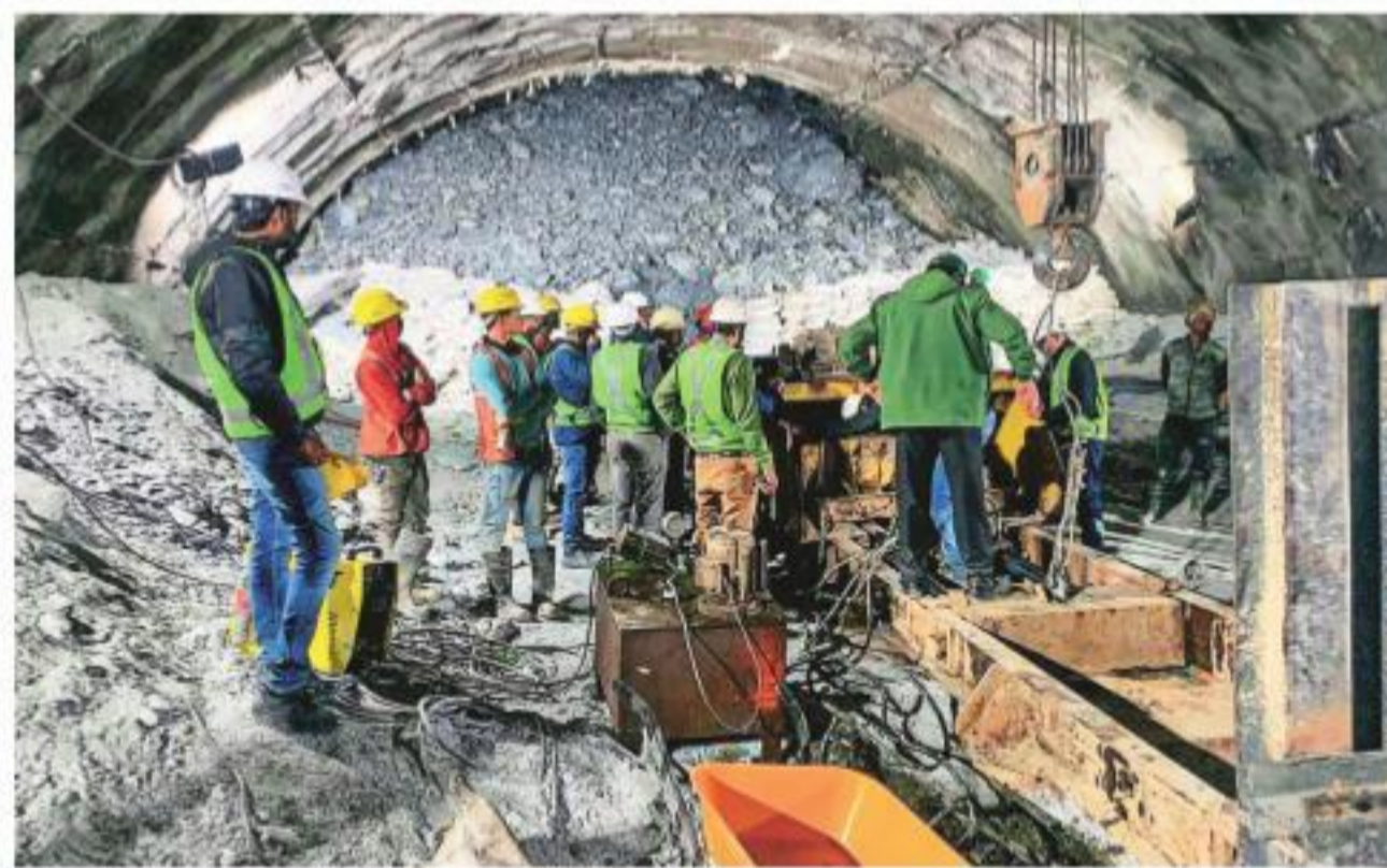
A part of the tunnel in Uttarkashi district has collapsed, walling up the passage. PTI
