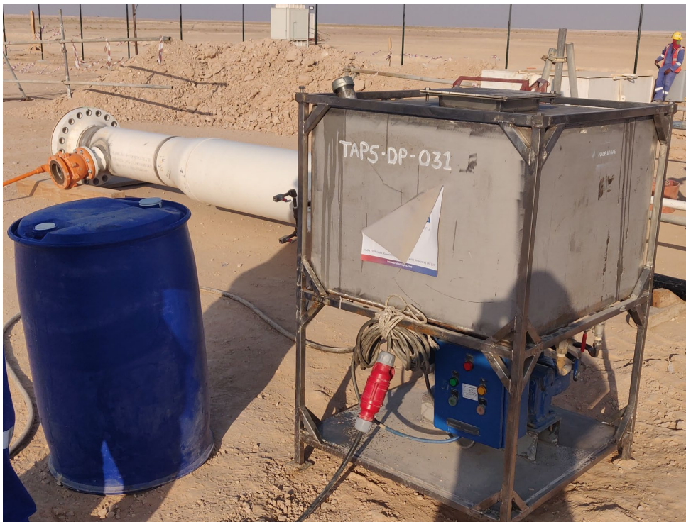
Corrosion inhibitor injection
