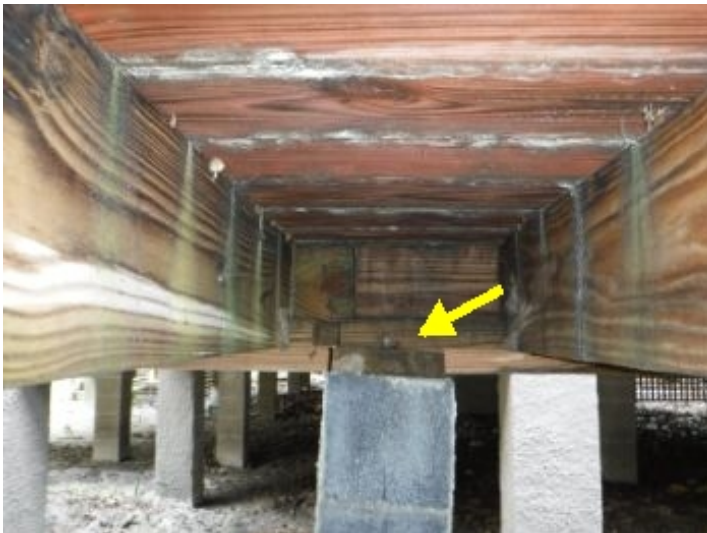
shows missing anchor bolts
