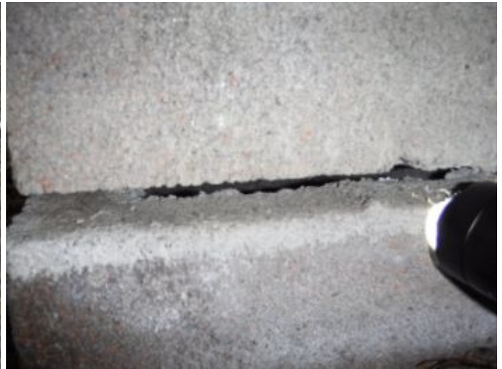
close up view of crack at bottom of pier reveals no reinforcing concrete or steel
