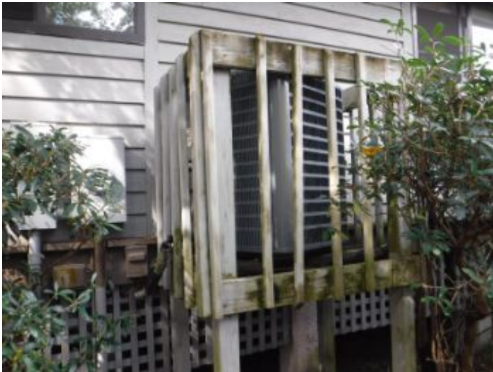
AC Support- Support deck is in need of minor repairs. Recommend improve.
