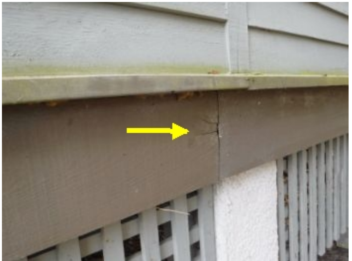
Decay (pictured)- Decay at pictured location. Repair as needed.
