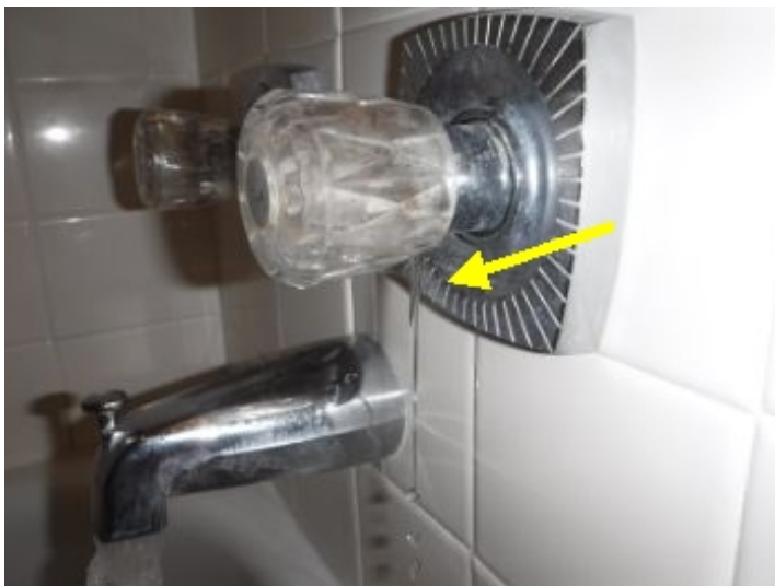
Faucet (leaks)- Faucet handle leaks while operating. Recommend contacting a licensed plumber to repair.
