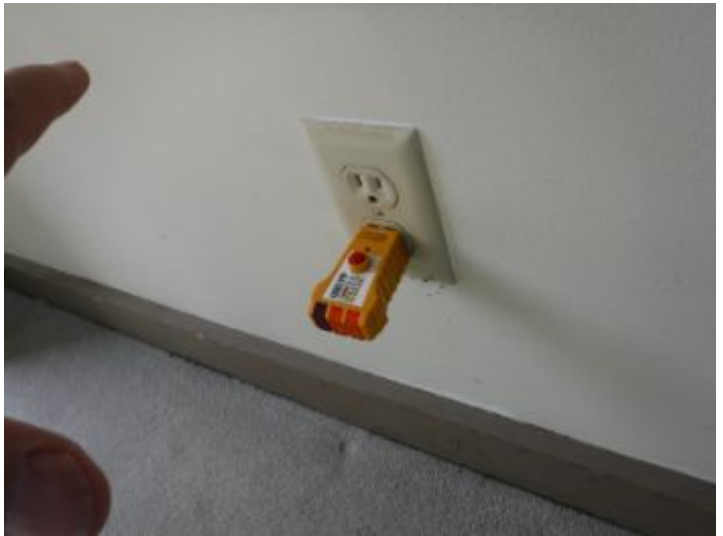
*Outlets- An electrical outlet/s as pictured showed an - loosely mounted in box - condition. Repair as needed. More than several noted.
