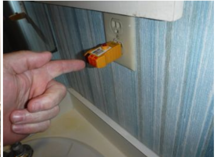
Not Protected- The bathroom receptacles did not test positive for GFI protection. Recommend improve for safety.
