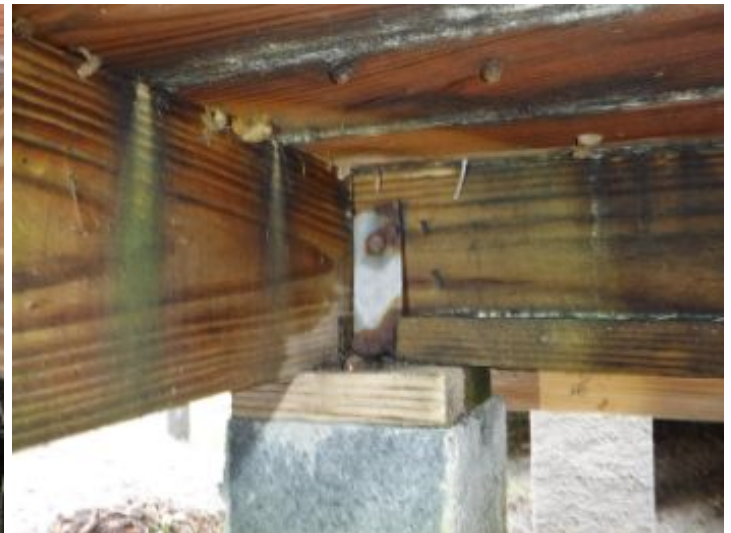
severely rusting anchor
