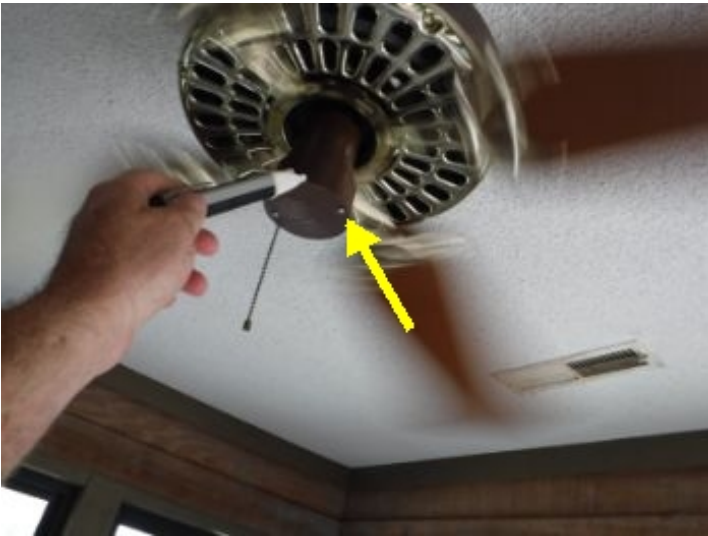
Tester indicated that some ceiling fans "may" be wired without a grounding conductor or has a grounding issue. While this test is not definitive we recommend checking one or two to be certain the grounding conductors are correctly fastened to the green grounding wire to the fan housing . Have a qualified electrician check this out for you.
