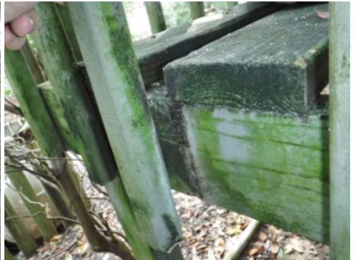
shows loose pickets on AC stand from rusting fasteners.
