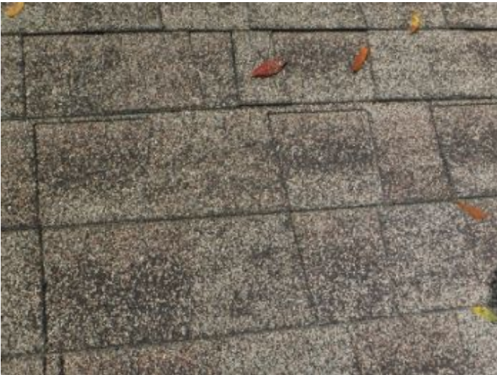
Granule Loss- Significant granule loss noted. Typically this is a sign that the roof covering is nearing the end of its useful life.
