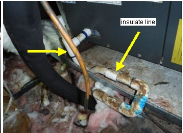
*Gunk or other buildup noted in the condensate trap. When traps clog a backup will happen. Recommend cleaning.
