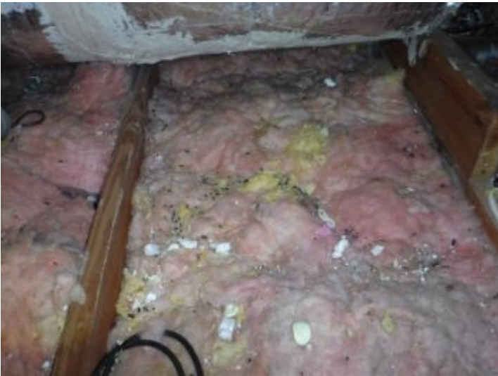
Rodents- Evidence of rodent entry into attic observed. Some insulation was noted with rodent feces on it. These should be replaced and attic should be reviewed for possible entry points.
