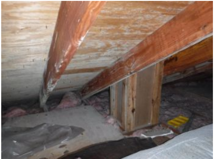
Microbial Growth- Some microbial growth observed on some framing components in the attic. Some areas are pictured. Although generally it was a modest amount it was not insignificant. Recommend improve attic ventilation. Some remediation is suggested (removal and treatment) especially if sensitive individuals.
