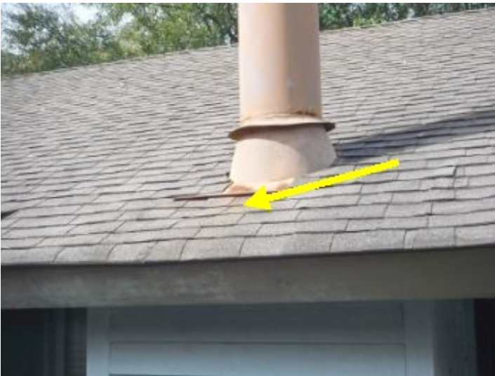
Area of concern- Area of concern pictured. - Probable leak under chimney area noted.
