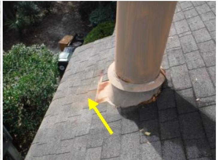
Area of concern- Area of concern pictured. - Probable leak under chimney area noted.
