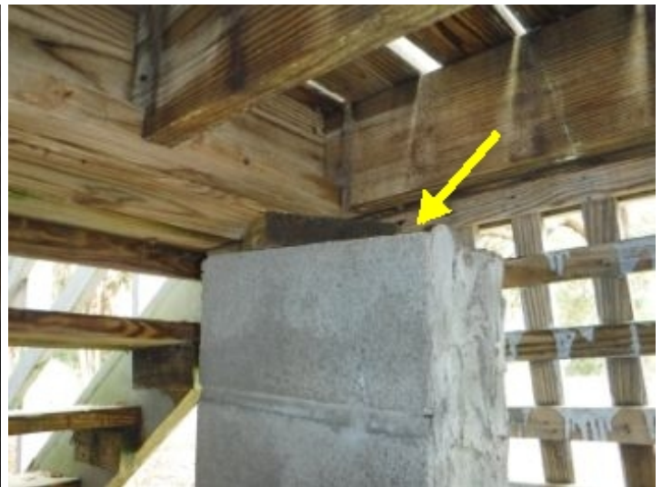
Pier by back deck stairs is leaning, is not filled with concrete and is open at top. Open cells are not allowed. Have it repaired.
