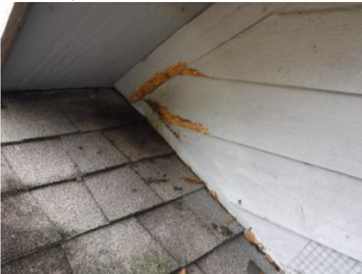
rodent chewed trim shown- improve flashing here at next re- roof
