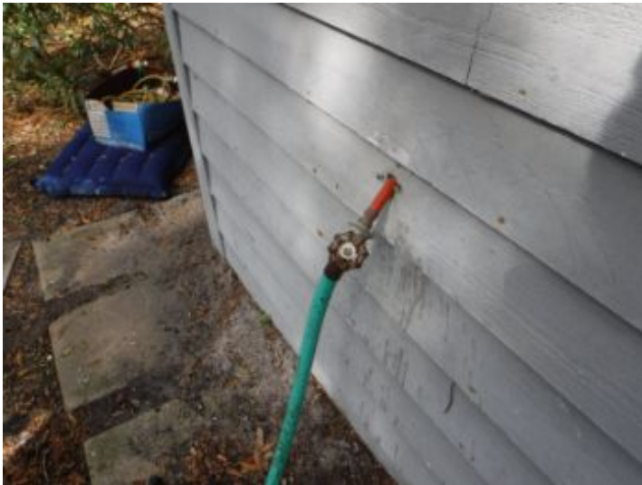
Hose bib (attachment)- Hose bib is not firmly attached. Repair as needed.
