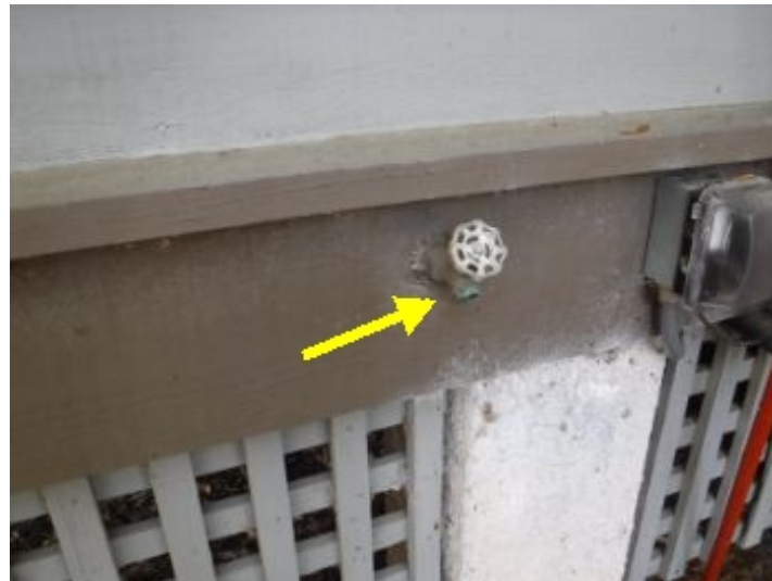
Absent (all)- Noted not present on hose bibs.(anti backflow devices) Recommend improve.
