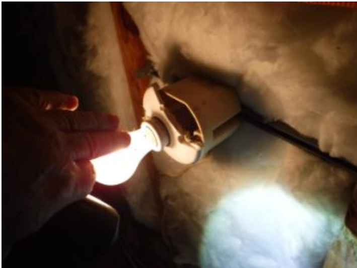
broken fixture needs replacement
