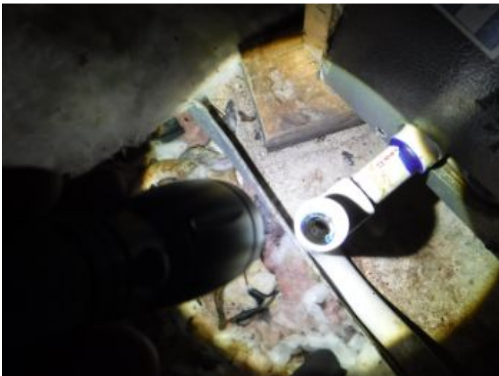
trap with cap removed showing gunk in trap- clean
