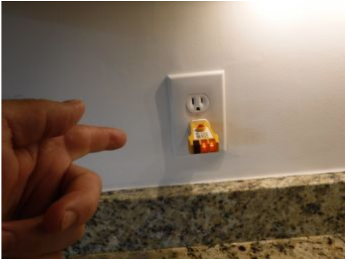
Not Protected kitchen- Some kitchen receptacles did not test positive for GFI protection. Modern rules specify all receptacles serving kitchen counters be GFI protected. Recommend improve for safety.
