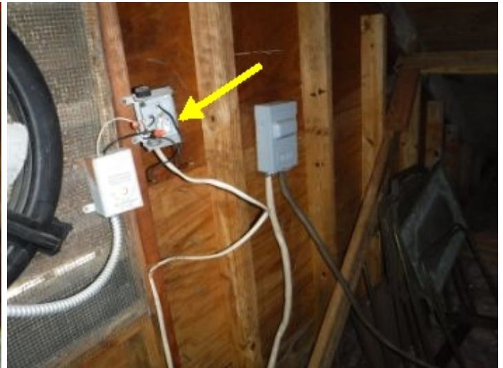
J Boxes, connections- Connections made outside of a junction box is not allowed and pose a safety hazard. Connections need to be made inside of a listed box with a suitable cover properly attached to framing as required. Recommend repair as needed.
