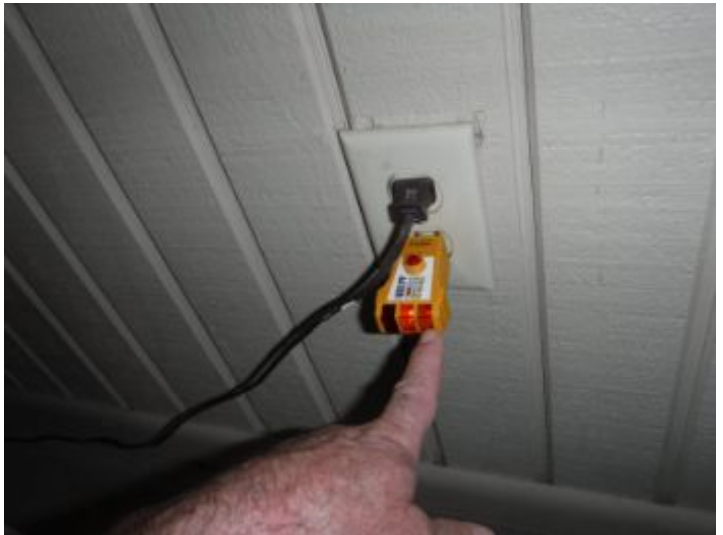
*Outlets- An electrical outlet/s as pictured showed an - loose connection - condition. Repair as needed.
