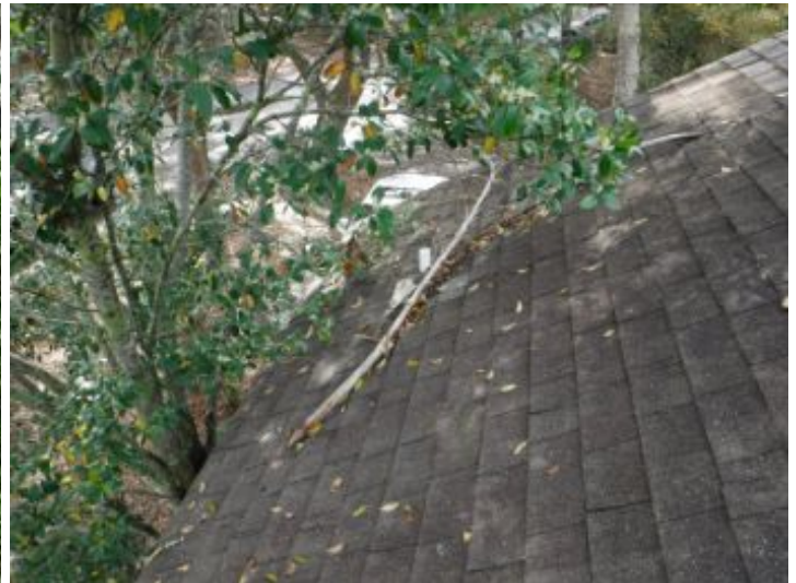
Maintenance suggestion- Leaves, pine straw and other debris should be swept off of roof regularly to protect the structure from moisture intrusion and prolong the life of the roof covering.
