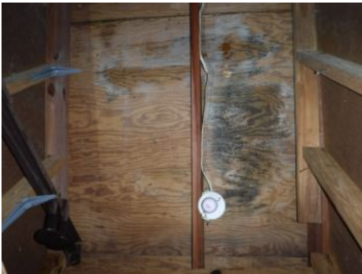
microbial growth on utility room ceiling- possible leak or insufficient ventilation in this area.
