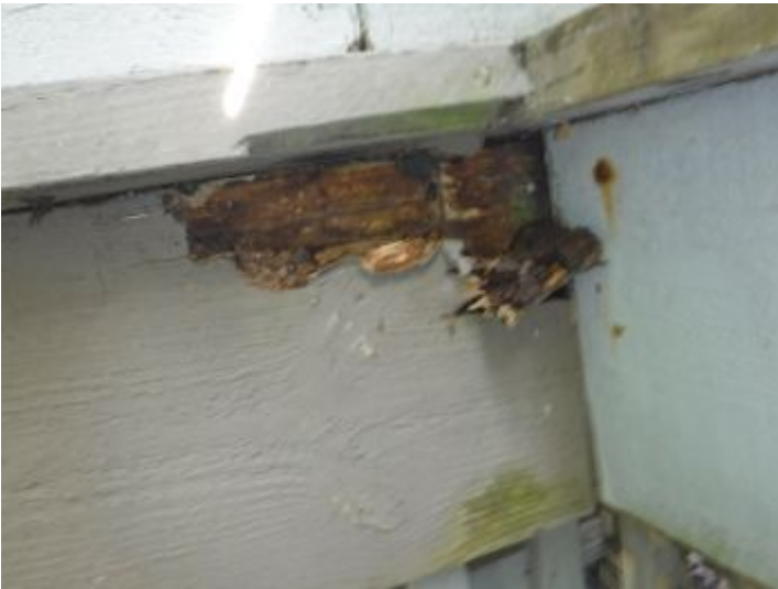
Decay (pictured)- Decay at pictured location. Repair as needed. In corner of deck.
