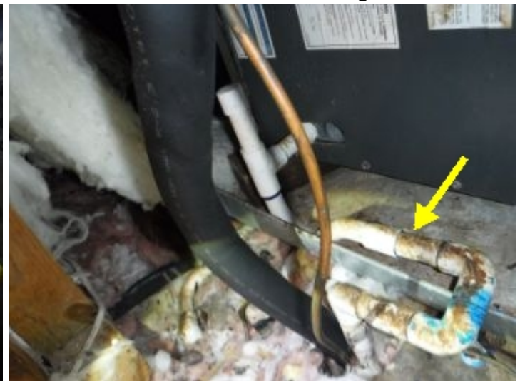
Insulation- Primary condensate line is not insulated. Line should be insulated in the attic areas to prevent condensation from forming on pipe. Condensation can damage building materials. Recommend improve.
