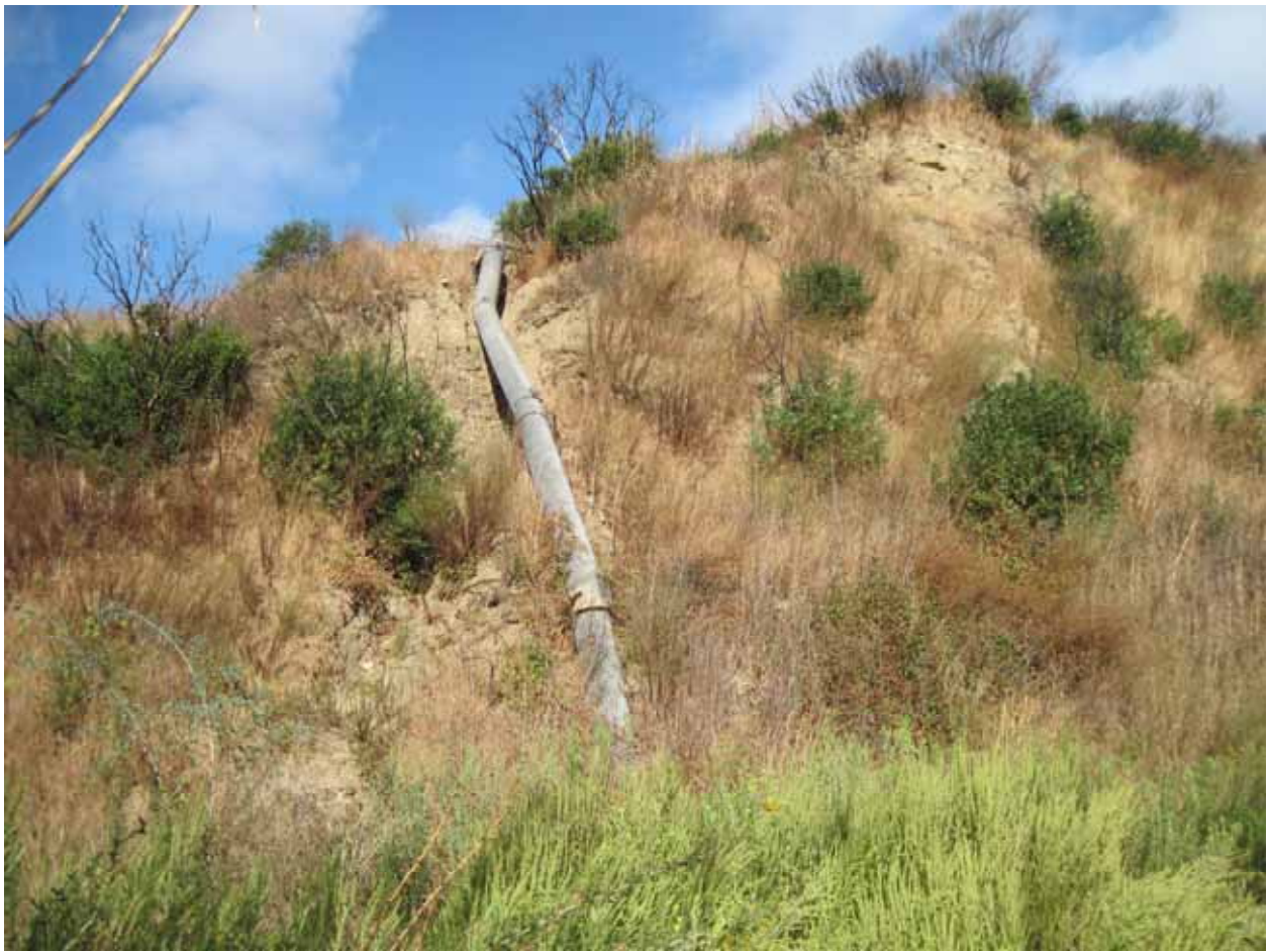
3. Stormwater conveyance pipe along the northern portion of the Subject Property.
