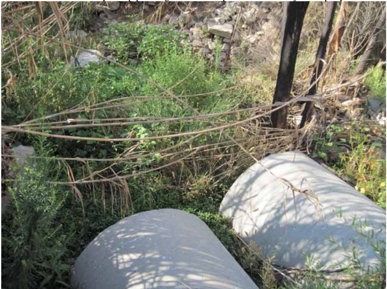
4. Stormwater control pipes within Carbon Creek.
