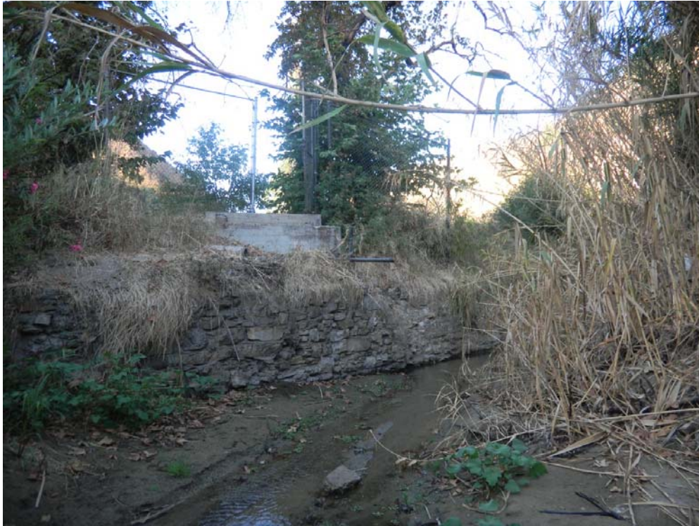
Photo 2: A few remnants of the La Vida resort. This photo shows an old retaining wall constructed to stabilize the creek bank. Concrete footings above the wall are for the footbridge (shown in Photo 1) that led from the bathhouse to the restaurant.
