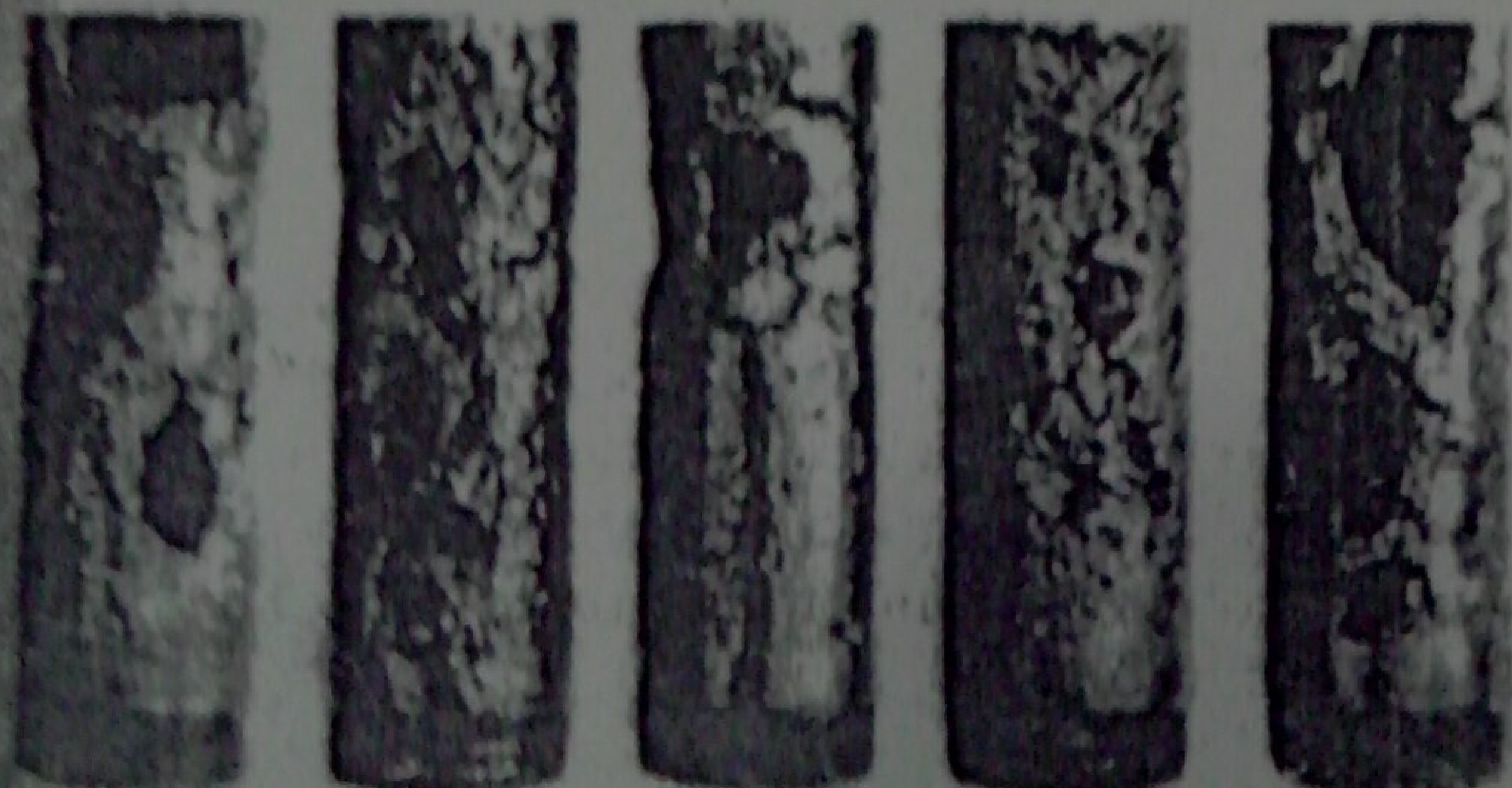
Figure 29-10. (A) Corroded cast iron pipes from a tidal marsh. Corrosion is due primarily to activities of sulfate-reducing bacteria. (B) Desulfovibrio sp. growing on an iron salts-agar medium. The colonies appear black because of iron sulfide formation. Desulfovibrio spp. occur widely in fresh, polluted, marine, and brackish waters. (Courtesy of W. P. Iverson and the National Bureau of Standards, U.S. Department of Commerce.)
