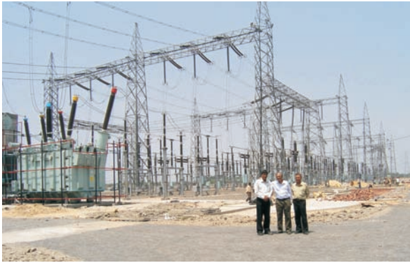
Chapter 15—Fig. 15.15 The substation of Powergrid Corporation of India (near Kolkata, India) where the FBG temperature sensors have been installed. In the photograph, the author is with Dr. Tarun Gangopadhyay and Dr. Kamal Dasgupta of CGCRI, Kolkata. Photo courtesy of Dr. Kamal Dasgupta and Dr. Tarun Gangopadhyay, CGCRI, Kolkata.
