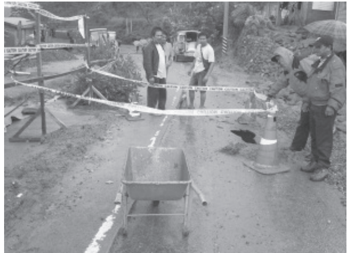
ROAD CUT: Combined elements from the City Disaster Coordinating Council led by Operation Officer Engr. Archiemor Ellamil put barricades and warning signs along a cut portion of road at kilometer 264 and 267, Marcos Highway during heavy downpour of rain caused by typhoon Julian last Wednesday. Marcos highway is closed for all vehicular traffic, kennon road is open only fro light vehicles while Naguillan Road is open to all type of vehicles.— By Bong cayabyab
