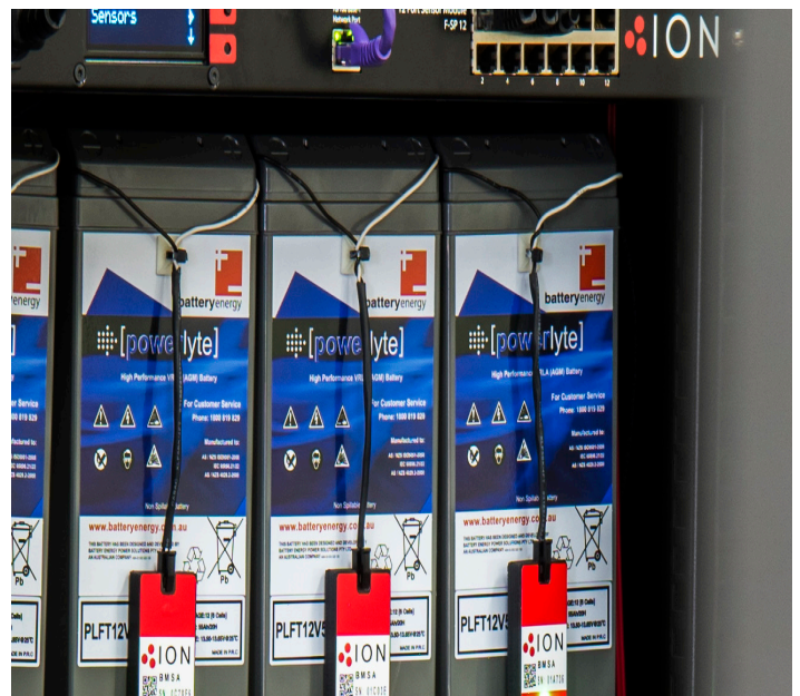
Three Battery Sensors installed and operating connected to front terminal batteries
