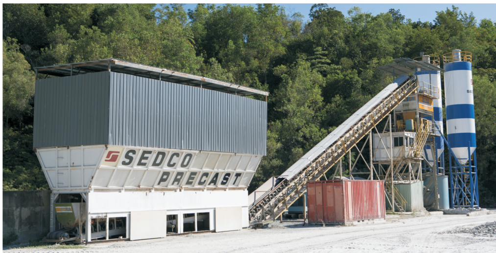
Batching Plant With Covered Hopper
