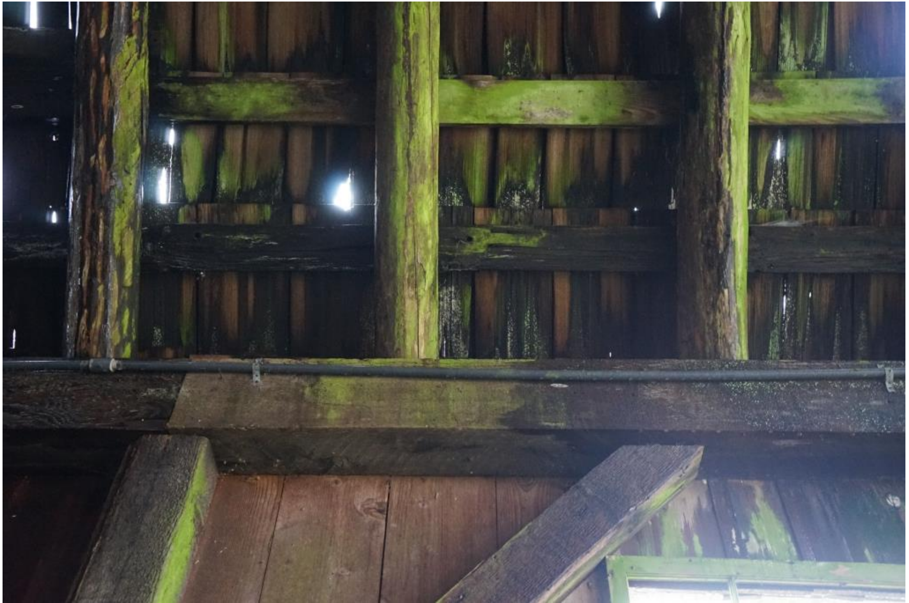
Detail showing connection of purlins to side wall plates, along with side wall posts and diagonal braces. All structural framing to be deconstructed and available for salvage.
