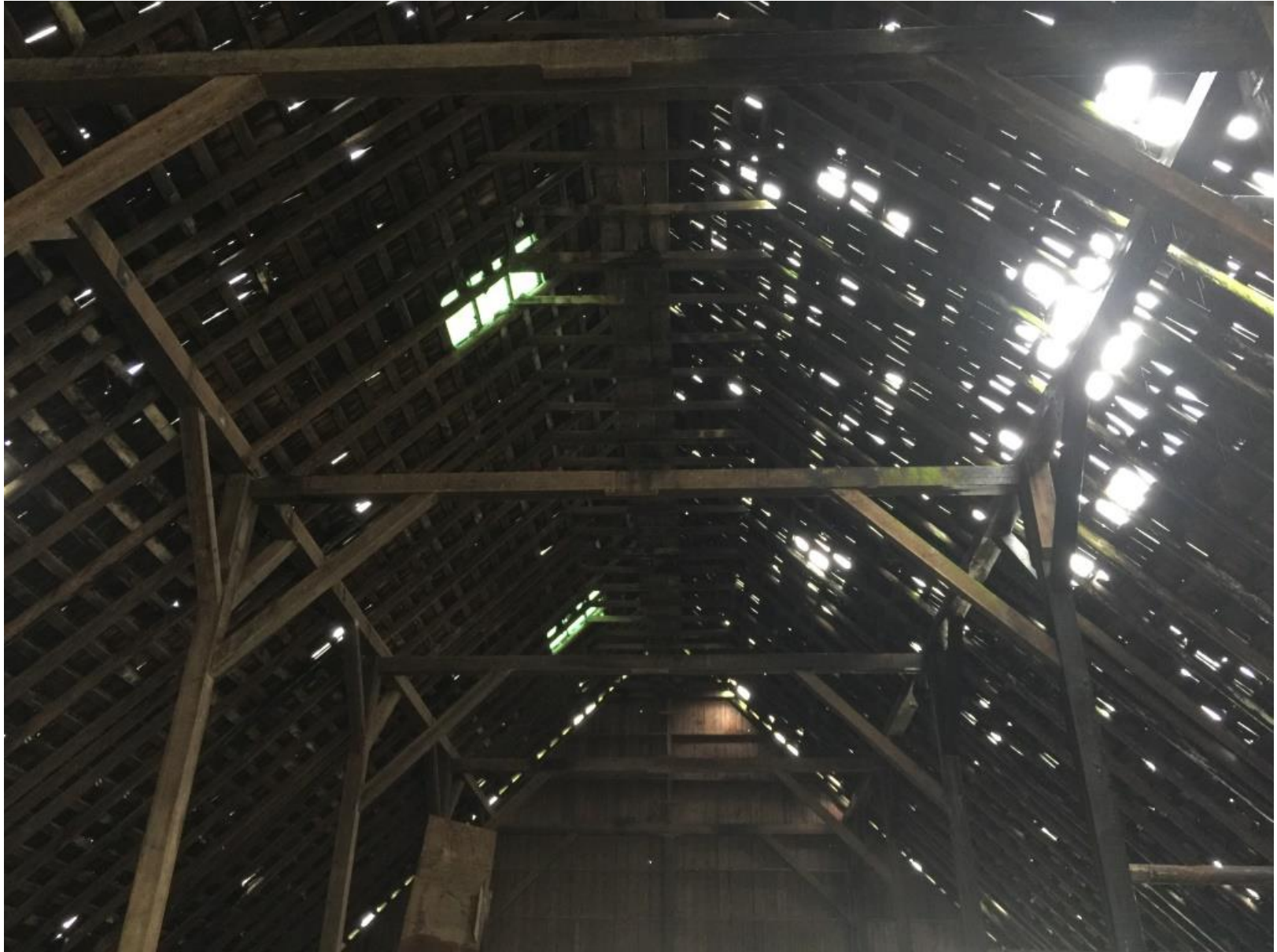
Image of structural system – all posts, beams, ties and braces to be deconstructed and available as salvage material.
