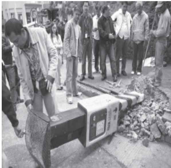
BAGUIO CITY -- Final Goodbye. City mayor Reinaldo Bautista Jr. (left) led city officials on Friday morning tearing down illegal structures along Session Road including some 6 P300,000-a-piece "unused" parking meters of the defunct Jadewell Parking Systems Corporation. Dispelling rumors that the controversial private parking system would do a comeback, Bautista Jr. who himself banned the parking firm from doing business in the city, led the physical tearing of the structures. --Ace Alegre
