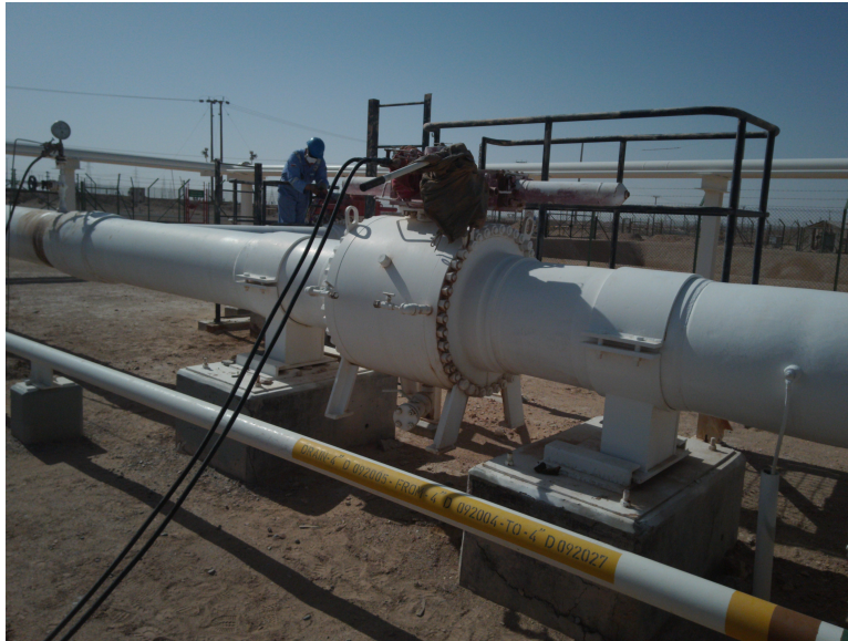
Figure 17: Closing main isolation valve using hydraulic pressure
