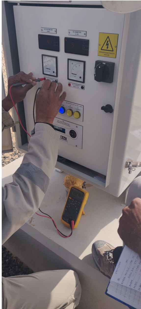
Figure 24: Measuring ON/OFF potential at transformer rectifier
