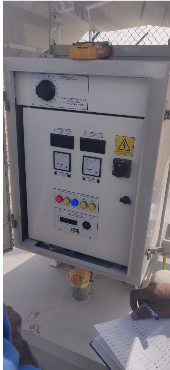
Figure 22: Cathodic protection transformer rectifier (inside)
