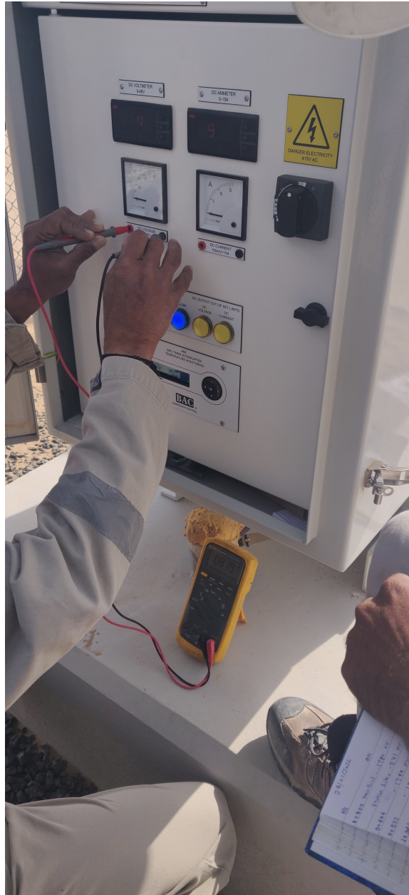
Figure 23: Measuring ON/OFF potential at transformer rectifier
