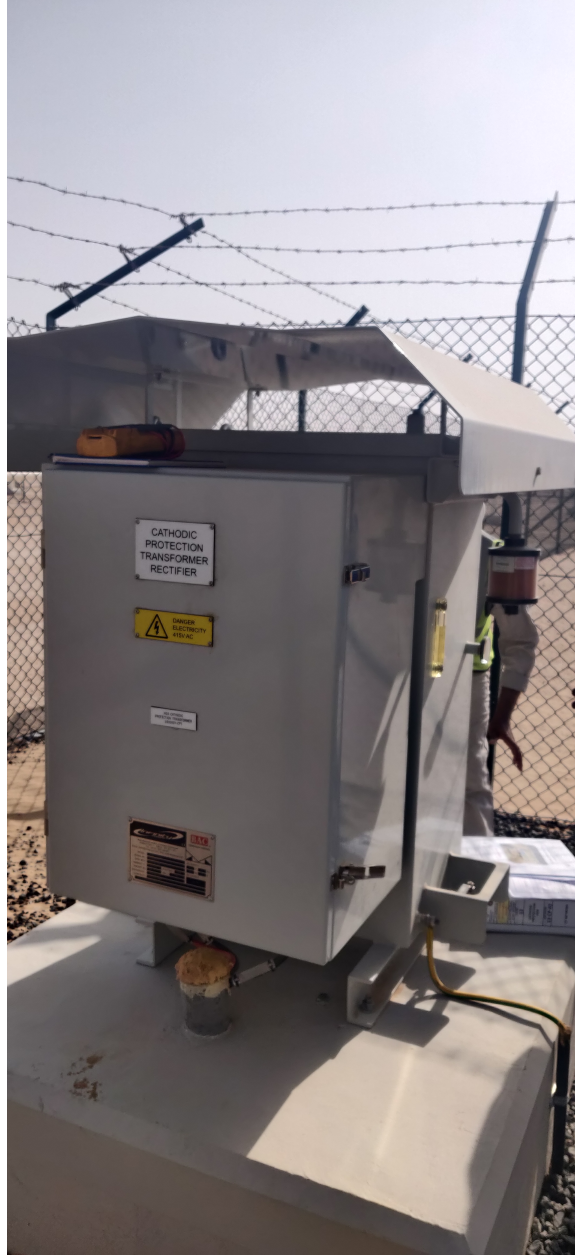
Figure 21: Cathodic protection transformer rectifier (outside)
