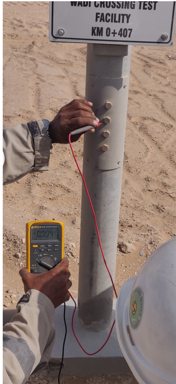
Figure 25: Measuring ON/OFF voltage
