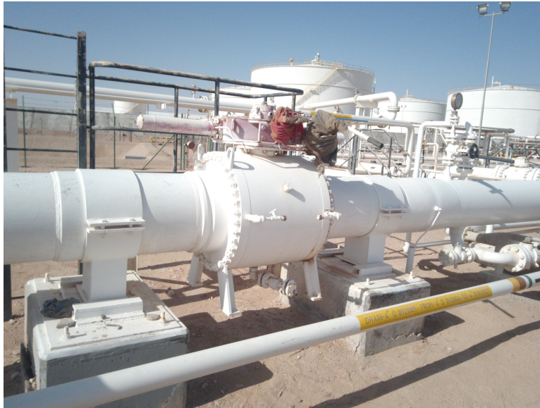
Figure 12: Main isolation valve 20" and drain 4"
